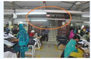
No backed up power emergency light has installed to illuminate the egress during emergency
