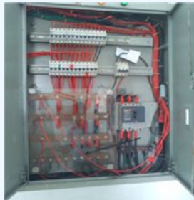
Haphazard cables in South-East DB of 2 nd floor
