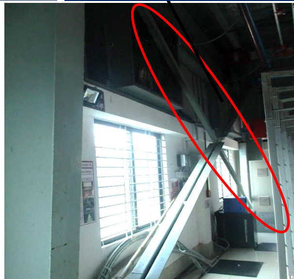
Single angle bracing was found instead of double angle bracing on south-west corner of 1 st floor
