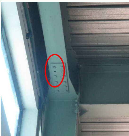
Missing bolts were found on edge column & beam joint on 1 st floor
