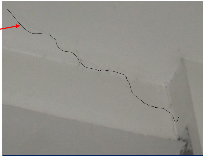
Crack on beam and landing slab
