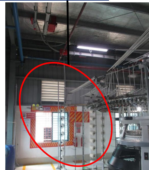
No vertical bracing was found at south-east corner of 1 st floor
