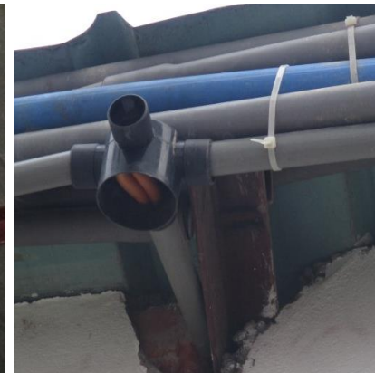
Steel roof angle was supported on edge by brick wall
