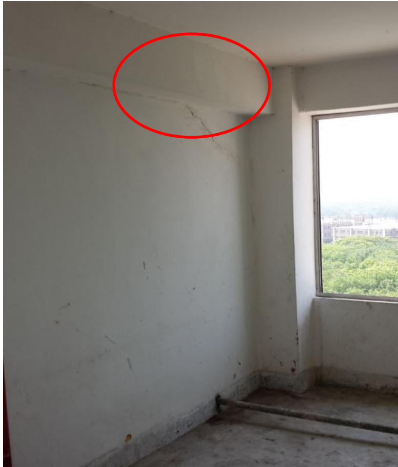
Penthouse Masonry Cracking
