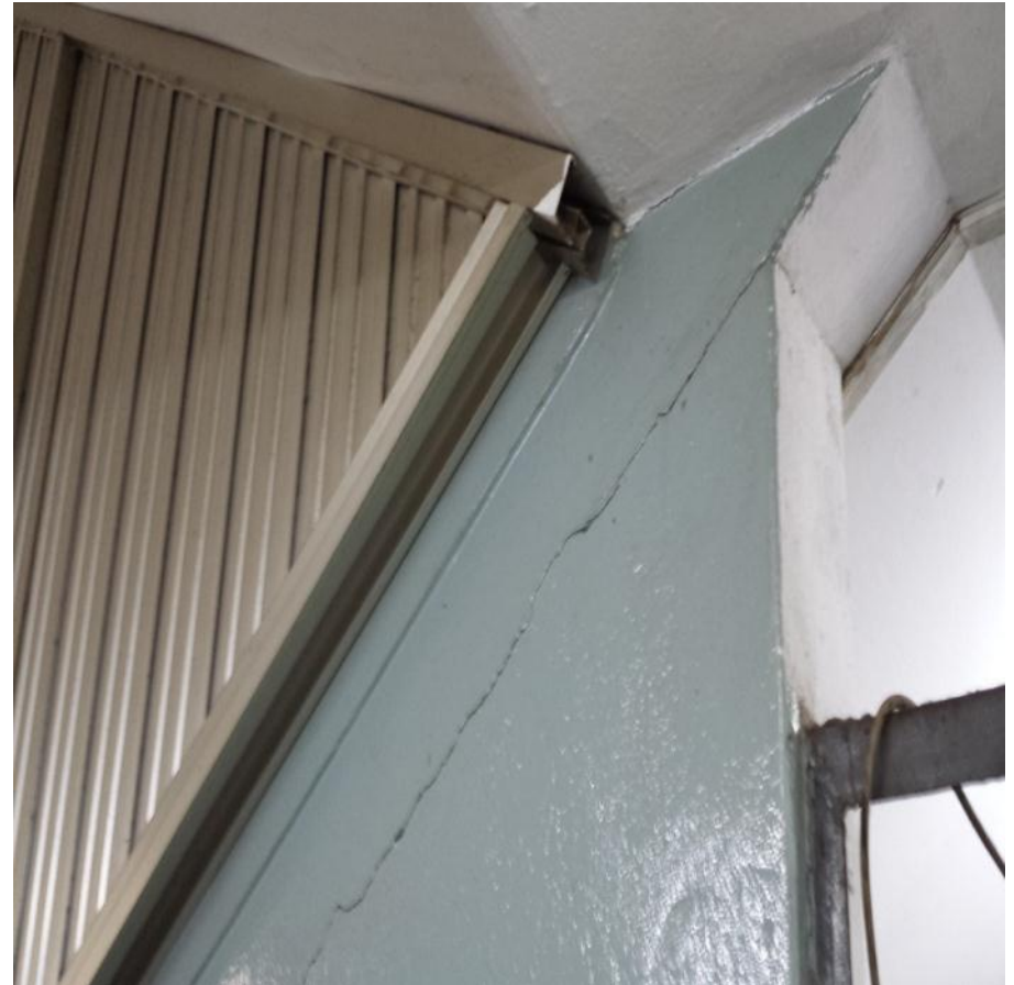
Cracking in stair-core Masonry
