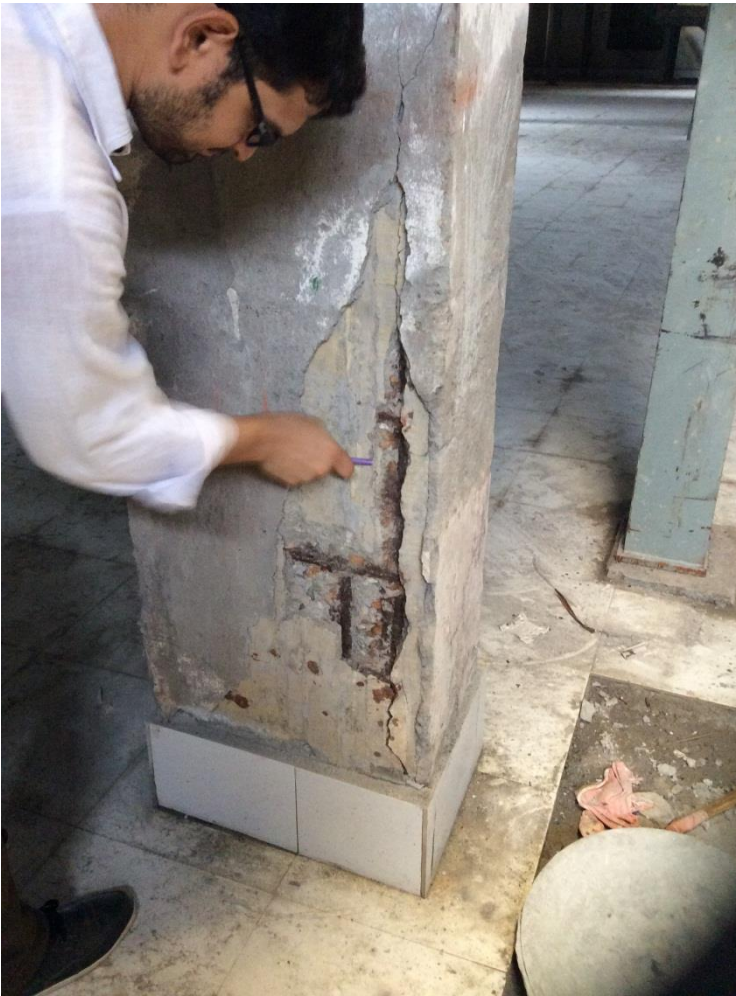
Corroded steel in concrete columns.
