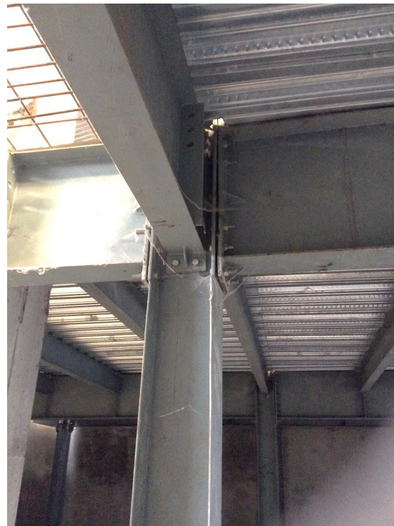
Large gaps between end plates and columns; generally poor connections throughout.
