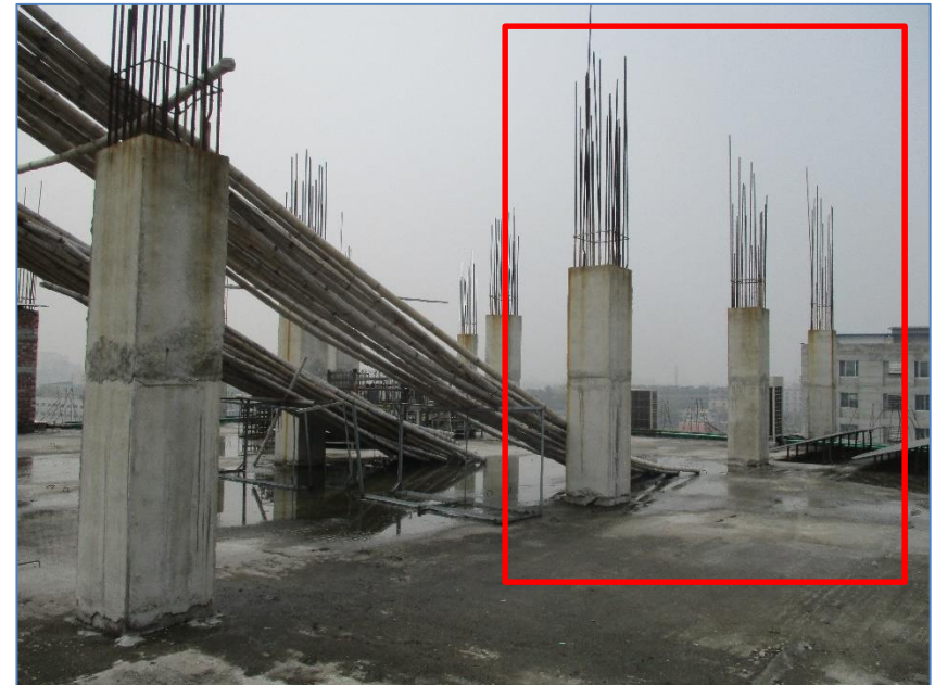
Exposed rebar on roof
