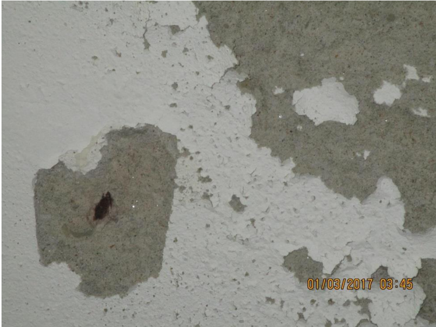
Corrosion on rebar due to dampness on roof slab was observed
