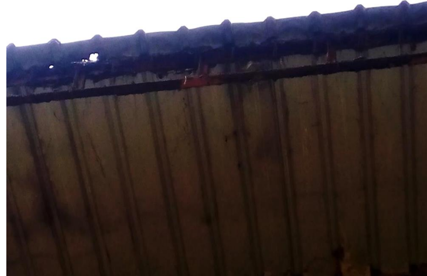
Corrosion on MS angle of truss member was observed
