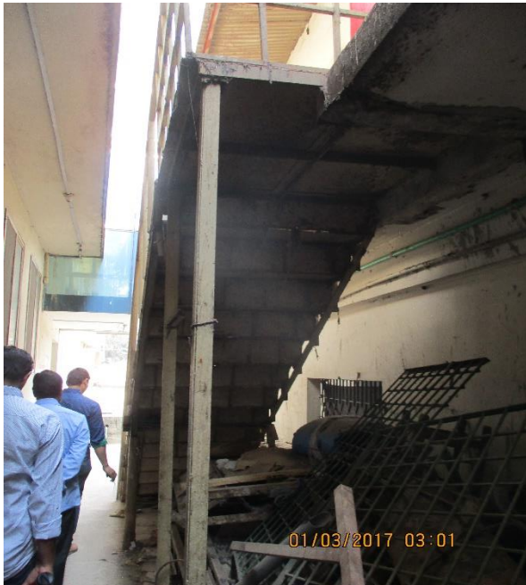
Apparently inadequate member sizes and thickness.
