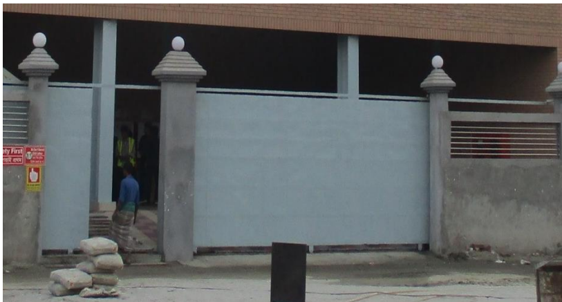
Wall bracing missing area in ground floor
