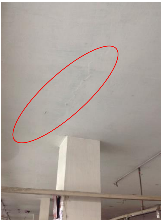
2 nd Floor soffit Crack on concrete slab soffit
