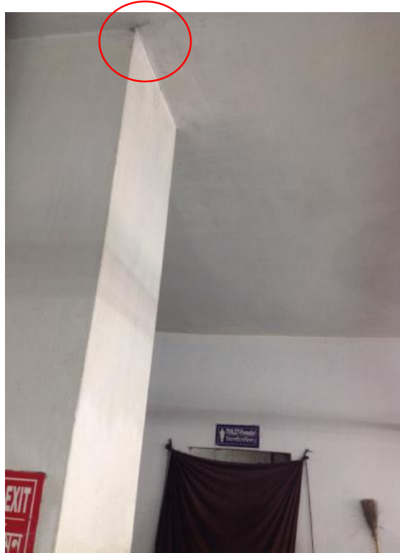
2 nd Floor soffit Crack originating from RC column
