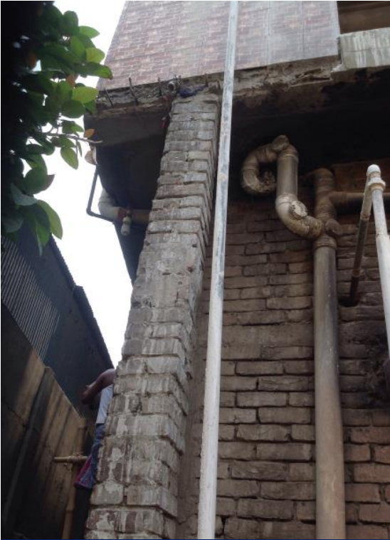
Ground Floor – External brick column is distorted/twisting.
