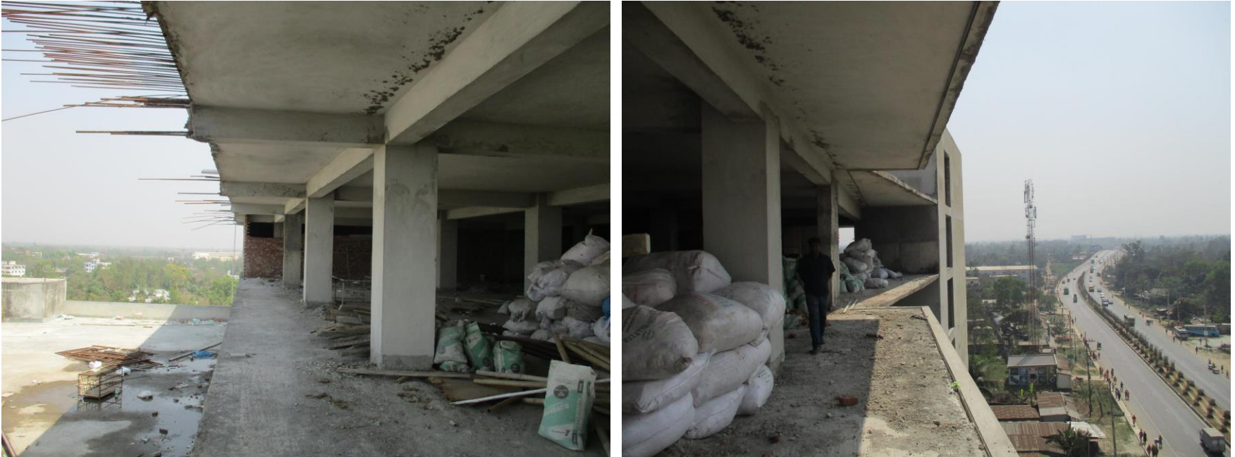
There are no edge protection around the floors which may causes falling hazard.
