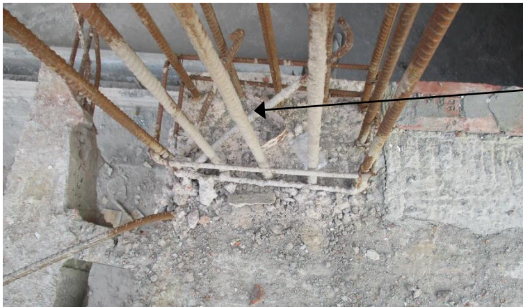
Exposed rebar of the Additional column
