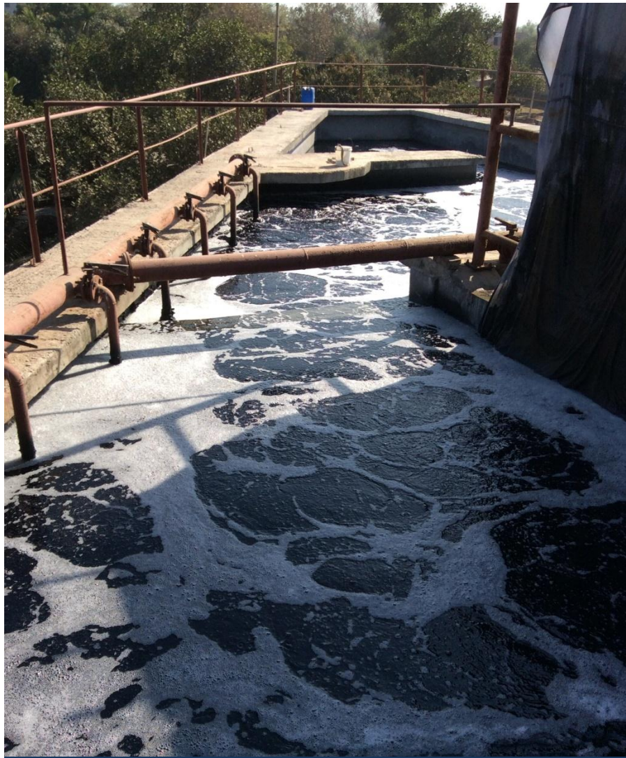
Edge protection only in place to prevent falls off of the tanks but not into tanks
