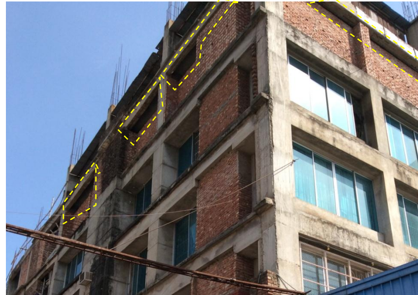
External masonry walls lacking top restraint
