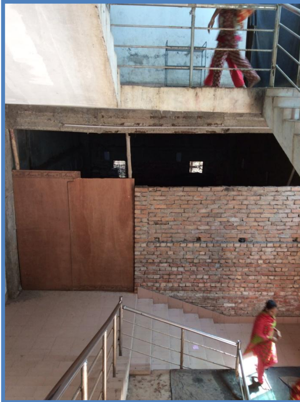
Internal masonry walls lacking top restraint
