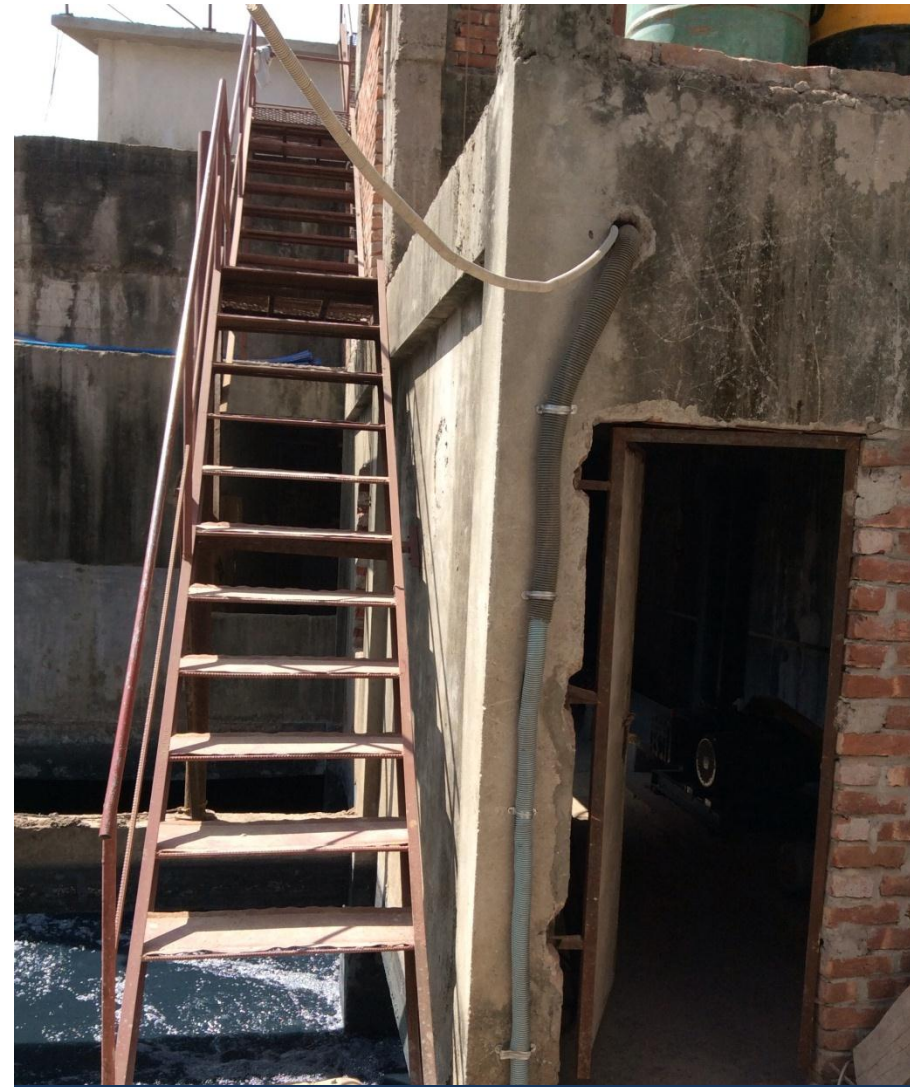
Apparently non-engineered stairs mainly fixed in place with welded reinforcement
