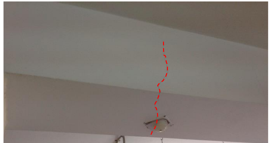
Hairline cracking to beam edges and soffits
