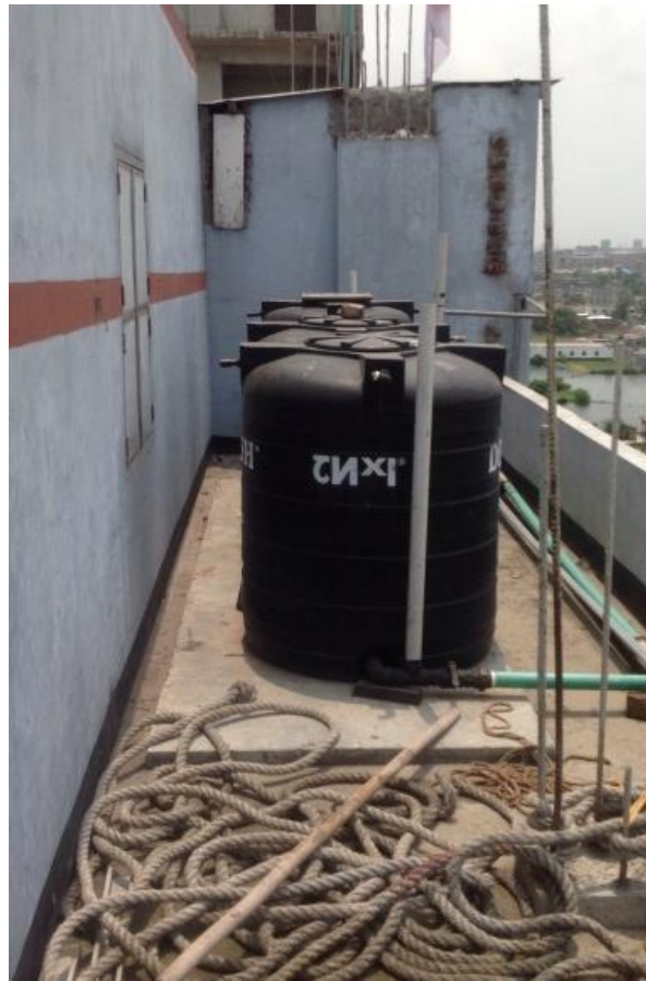
1000L capacity Gazi water tanks to Roof of Building 1
