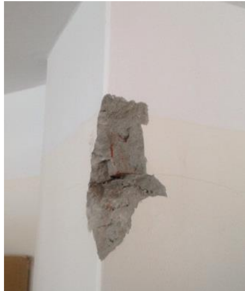
Exposed Column G.L. E / 2
