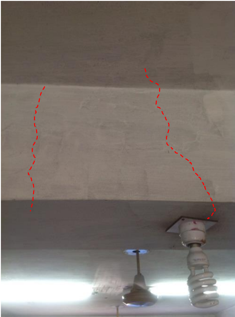
Hairline cracking to beam edges and soffits
