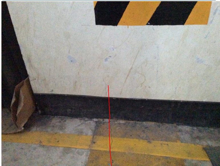
Cracking on ground floor adjacent to column
