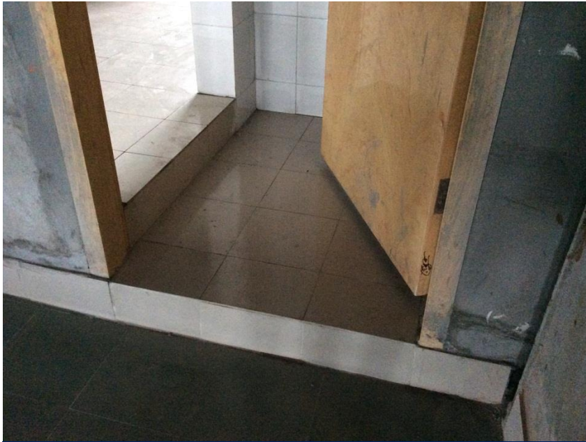
Heavy loading from toilet plinths 210mm+170mm
