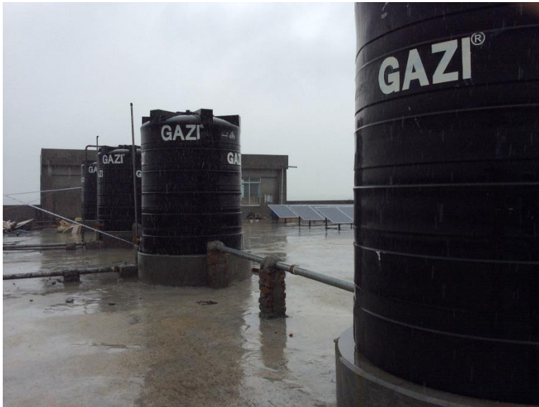
4 x 5000L water tanks with 485mm build up
