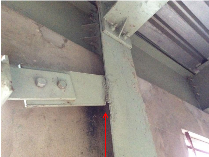
Poorly welded bracing onto column
