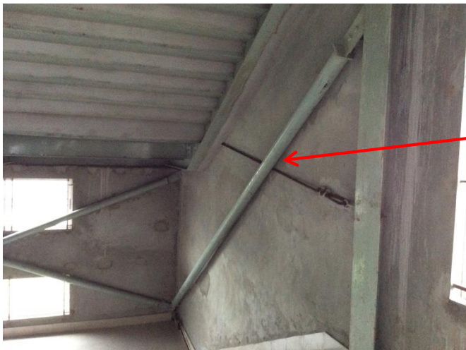
Typical bracing system - Tie not connected to column node
