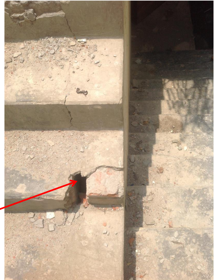
Cracking of stairs
