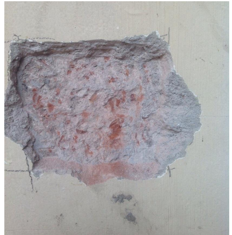
Brick aggregate was observed on site.
