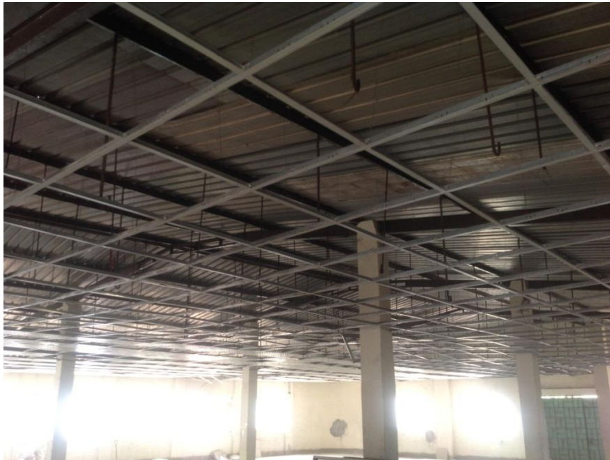
No roof trusses were observed in the Shed 2.
