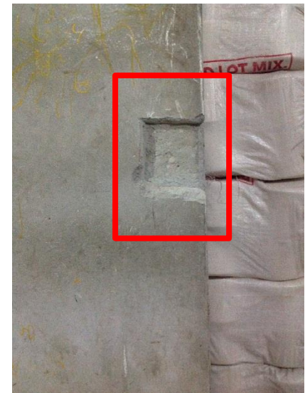
Tested Ground Floor Column – Stone Chips
