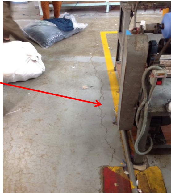
Crack over ground tie beams
