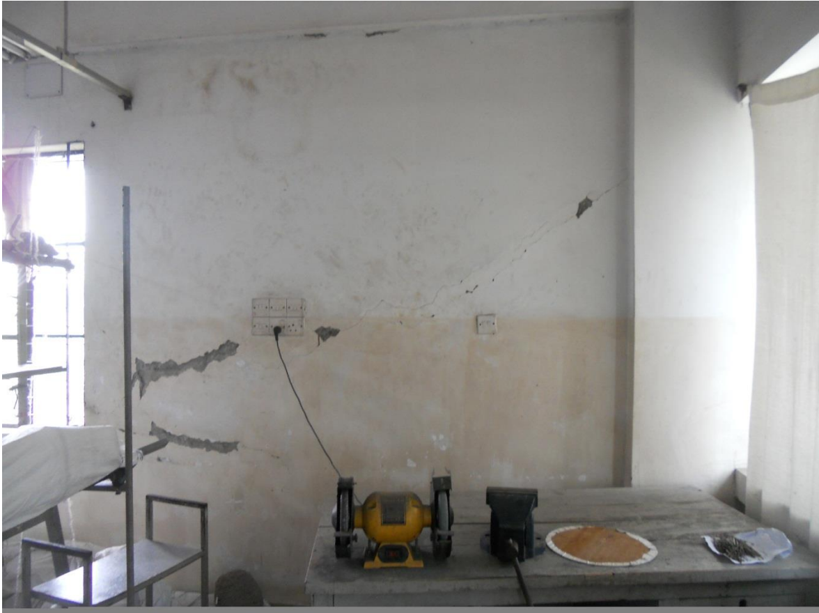
Cracking in masonry at West end of building
