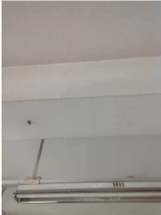
Hairline crack in beam
