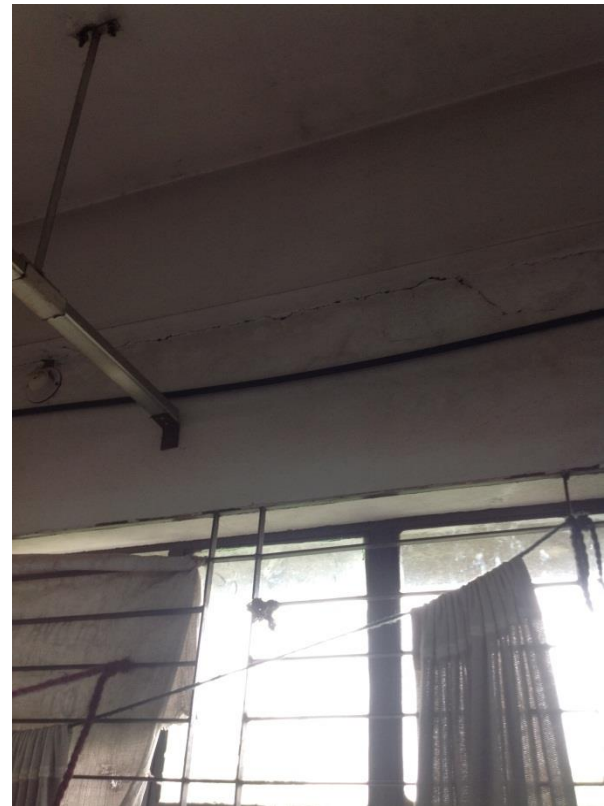
Cracking along edge beams
