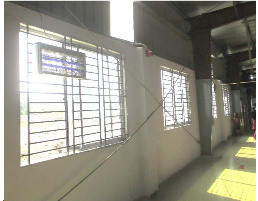
Loose vertical bracings
