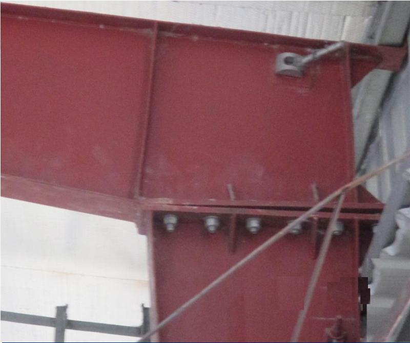
Gap at rafter & column connection
