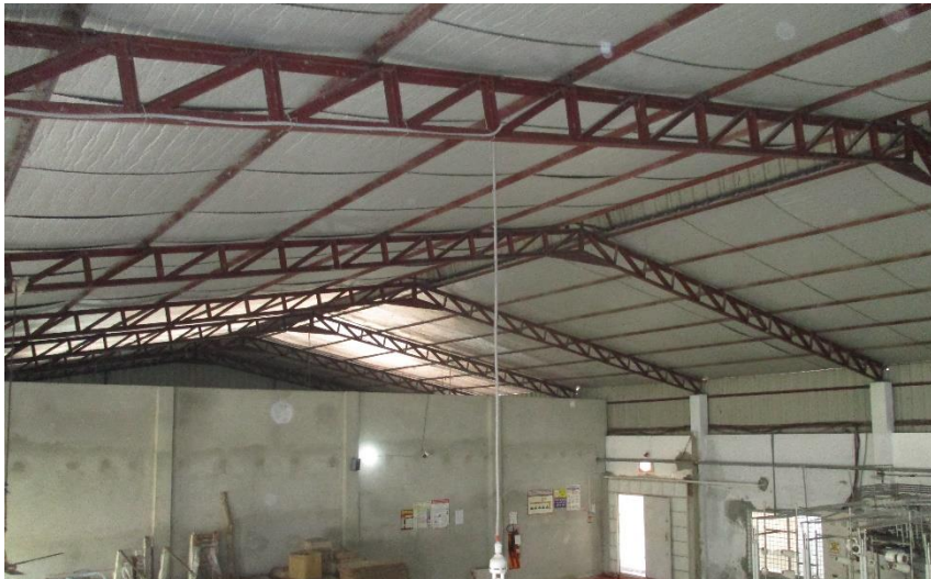
No lateral system were observed to resist lateral loading.(Shed#1)
