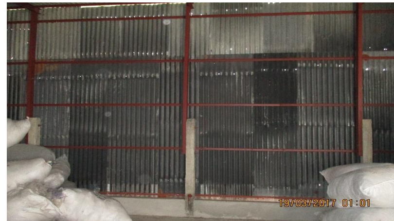
Non engineered connections (Shed#3)
