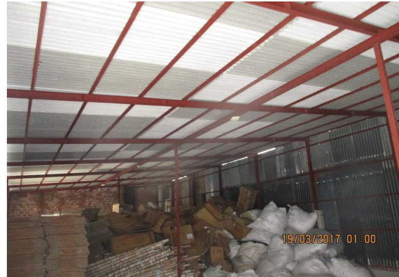
Apparently Non engineered (Shed#3)
