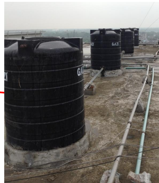
4 no. plastic water tanks
