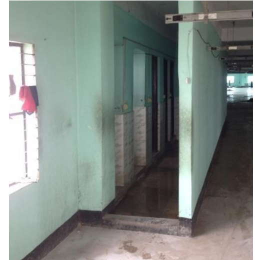
Typical toilet block
