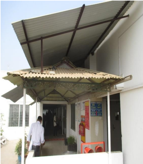
Non engineered canopy at 8 th floor level
