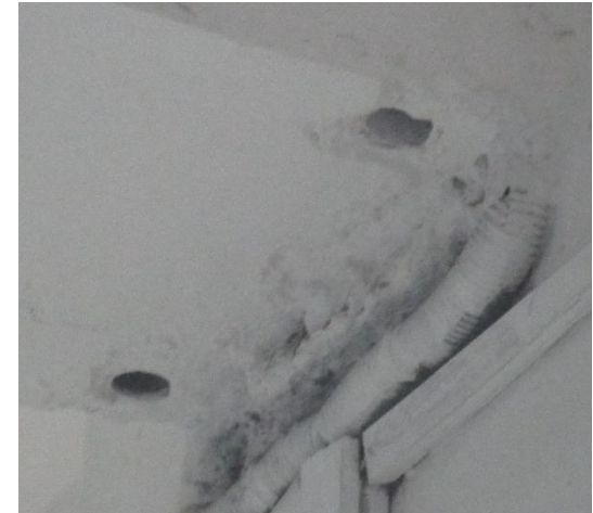
Hole on shear zone at 4 th floor
