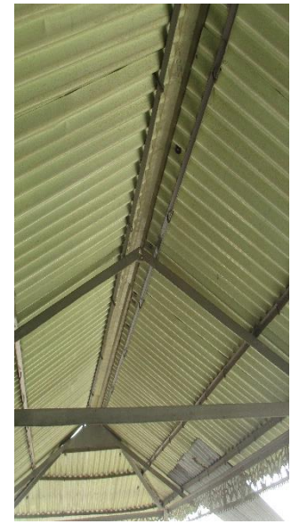
Non engineered connection of shed on 8 th floor
