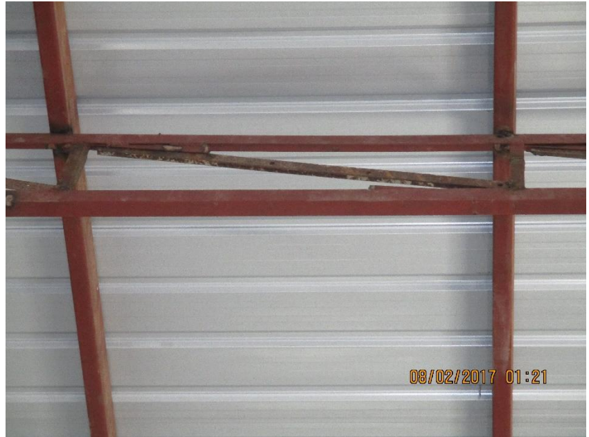
Defected structural member-Boiler shed
