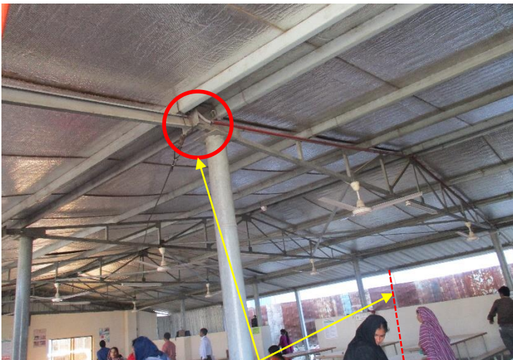
Poor connection -Dining shed
