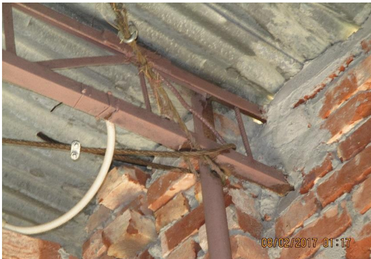
Poor Connection Details-Wastage storage
