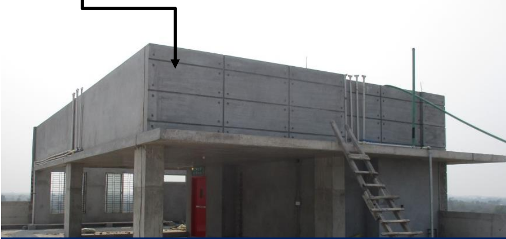
Found single RCC over head water tank on stair case
