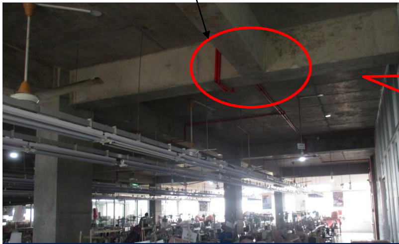
Crack observed on the joint of two beam
