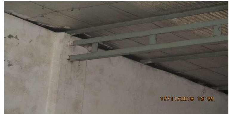
Non engineered connection (Fabric Storage, Production Shed)
