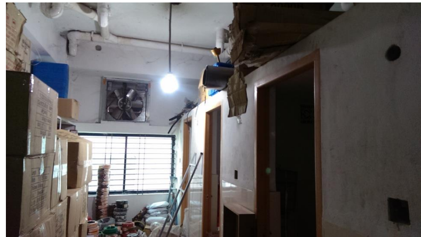
Additional storage loading on the 1 st floor.
