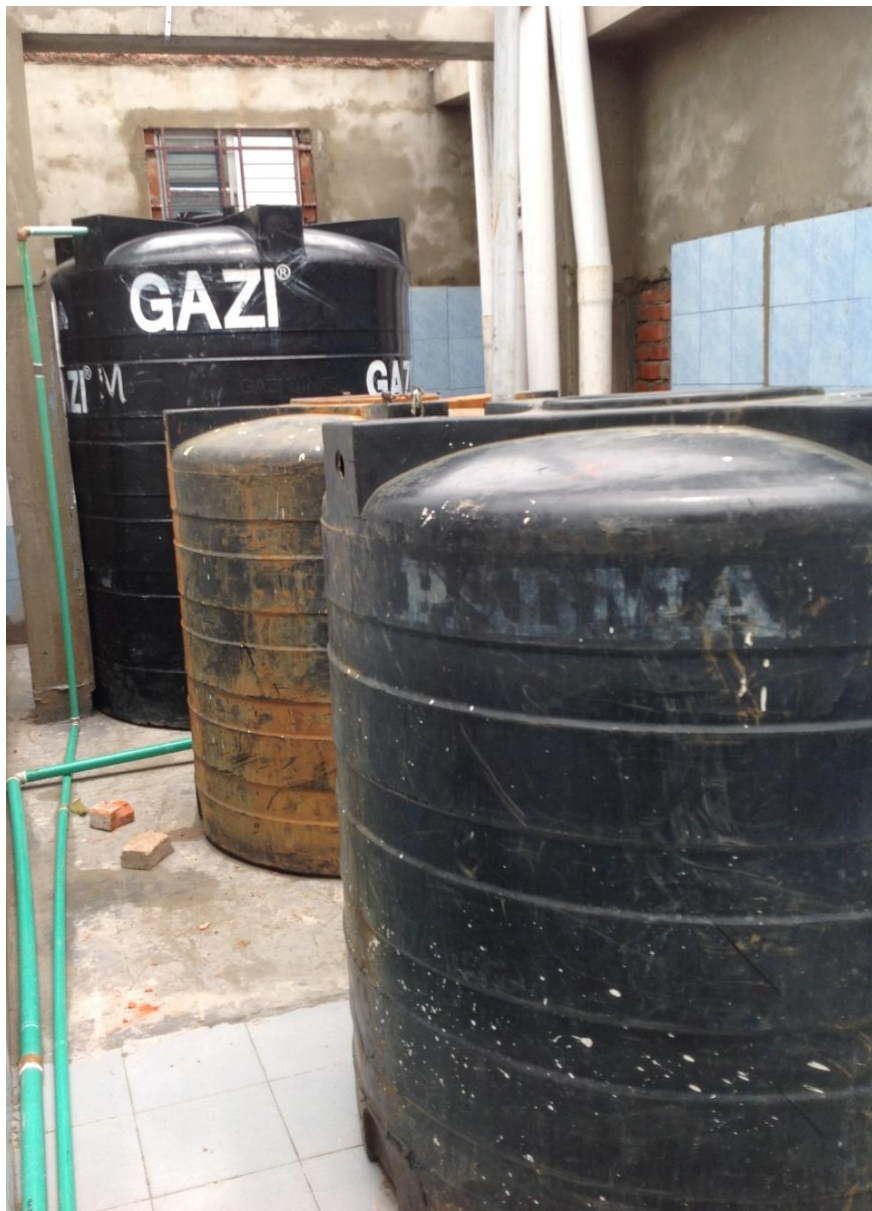
2,000 to 5,000 litre water tanks at 4th floor level
