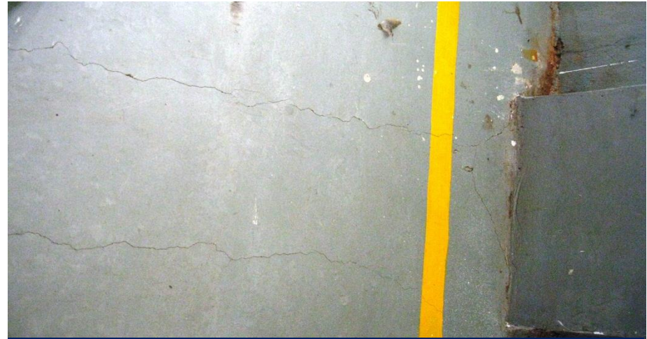
Cracking to top of slab
