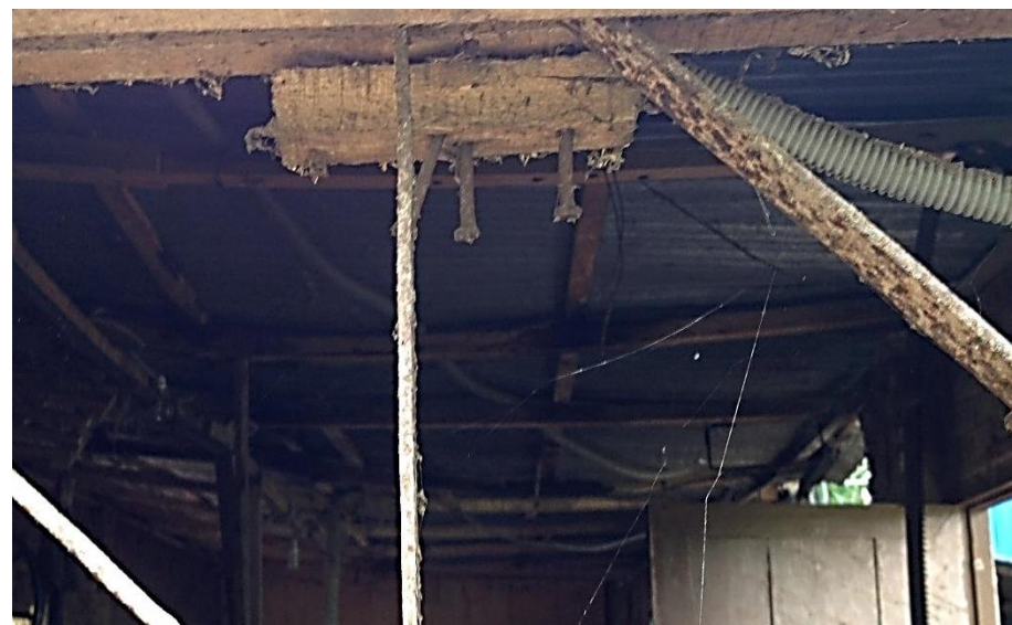
Wastage store – Sagging timber purlins
