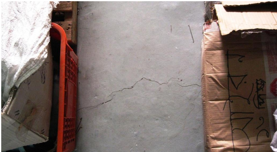
Cracking to top of slab
