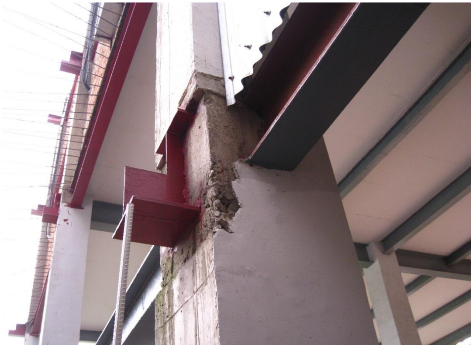
Rigidity of RC column to beam connection is not clear
