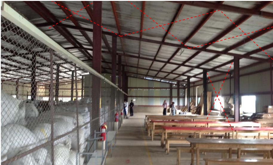
Roof shed - lack of horizontal bracing
