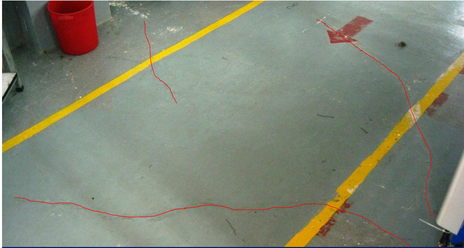
Cracking to top of slab
