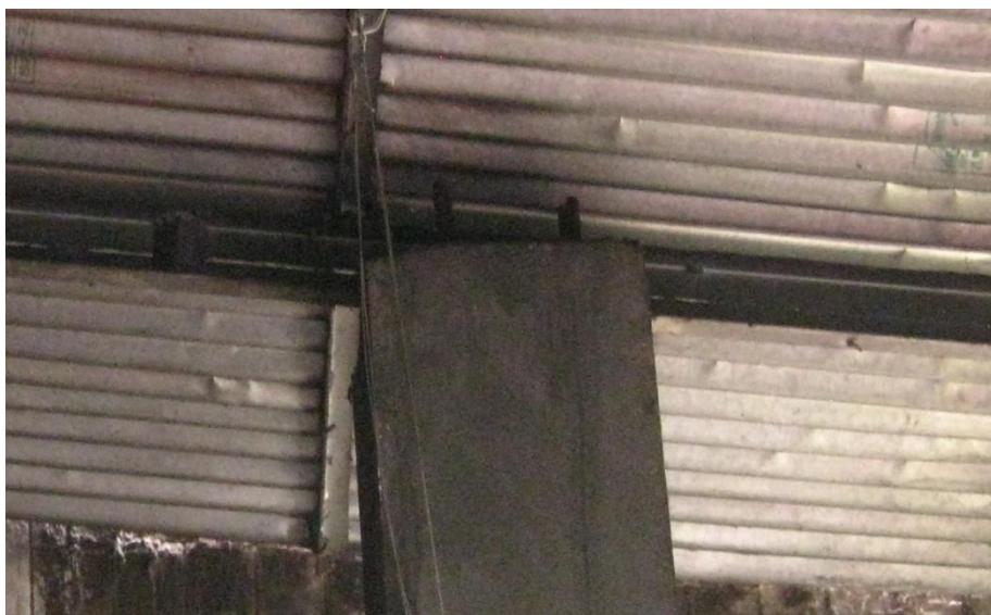
Generator Shed – Roof connection details unclear
