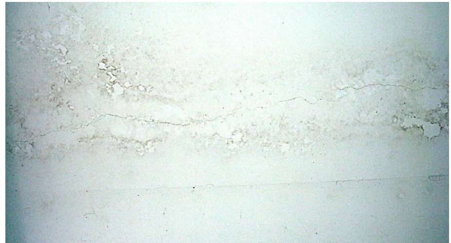
Cracking to soffit of the slab
