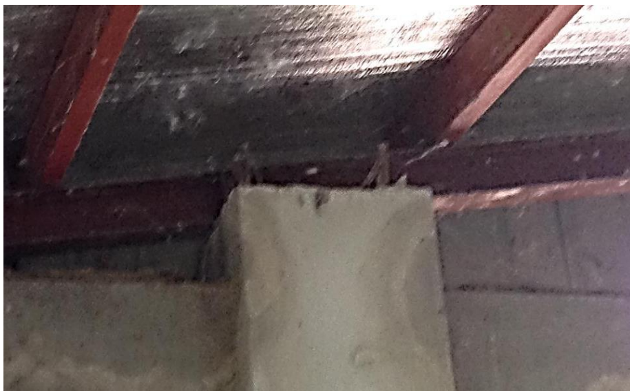
Shed to roof – Beam to RC column connection unclear
