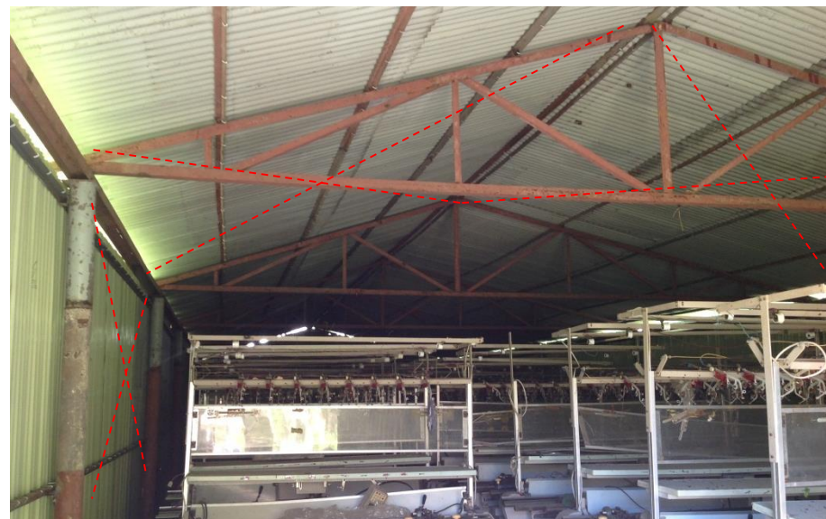
Store Shed – Lack of horizontal and vertical bracing
