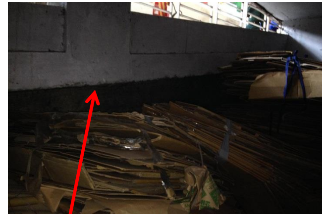
Column built off edge of ramp slab (support?)
