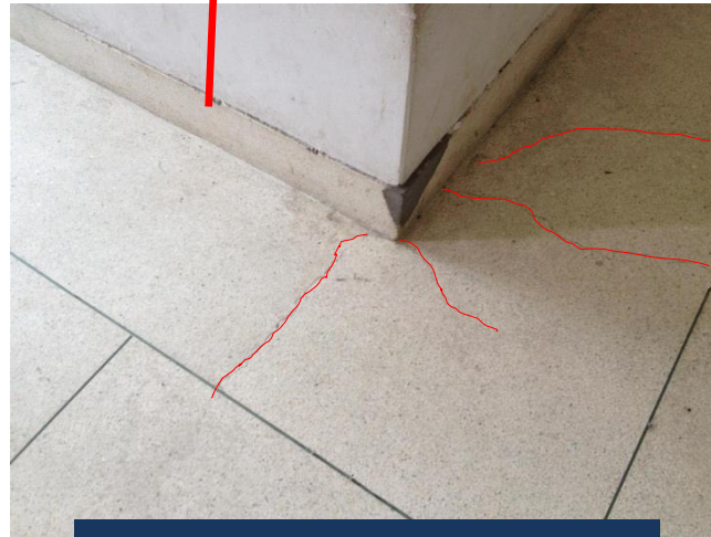
Cracking to ground floor slab.
