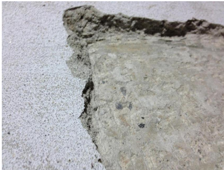
Tested Basement Floor Column – Stone Chips
