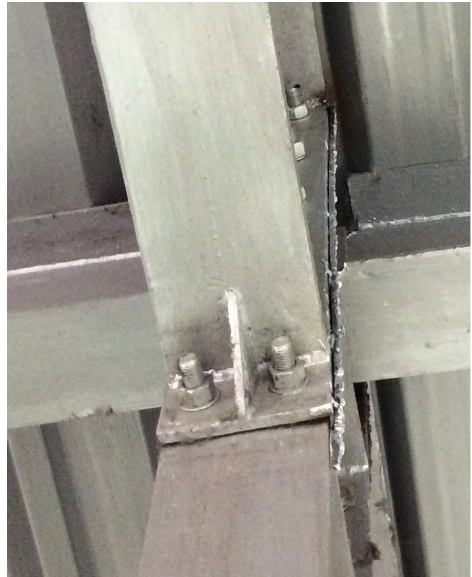
Shed 1 – In many cases where rebar appears to have been welded to end plates as a remedial solution to inadequate bearing, the detail is poorly executed.
