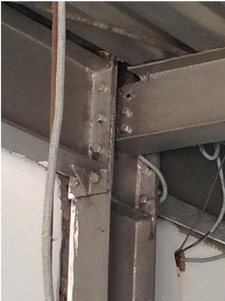
Shed 1 – Missing bolts
