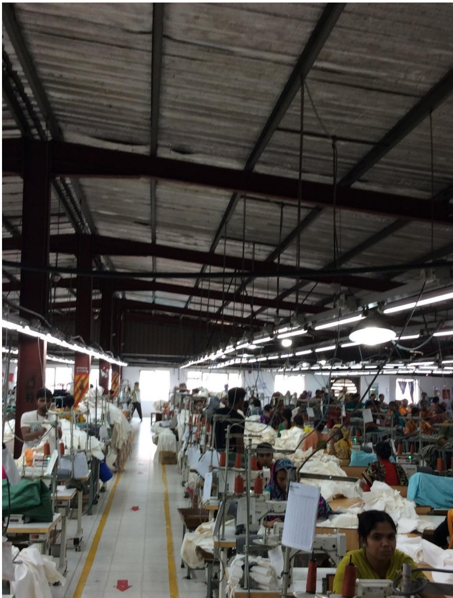
Shed 2 – Two-storey structure – Horizontal and vertical bracing missing
