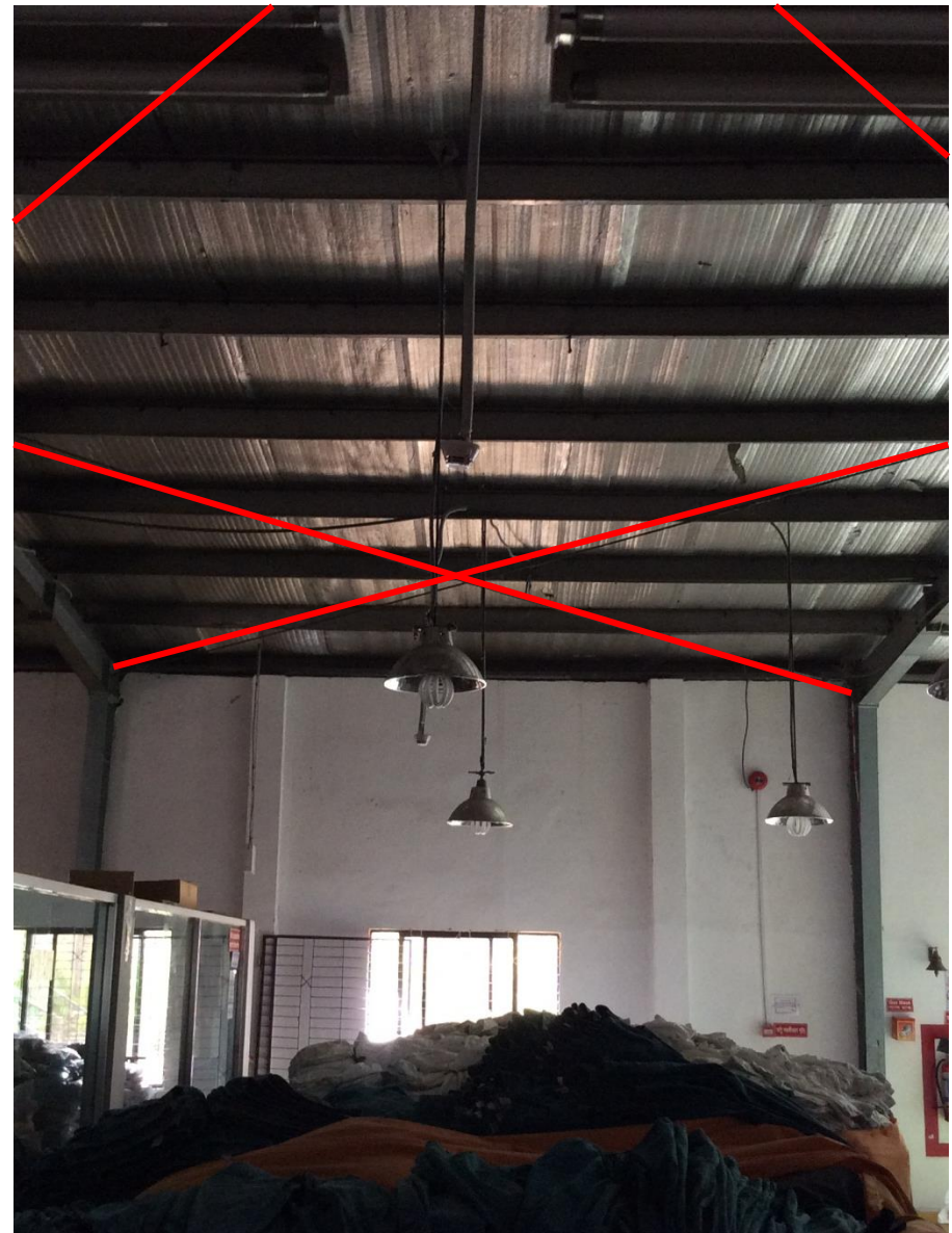
Shed 2 – Single-storey structure – Horizontal bracing missing
