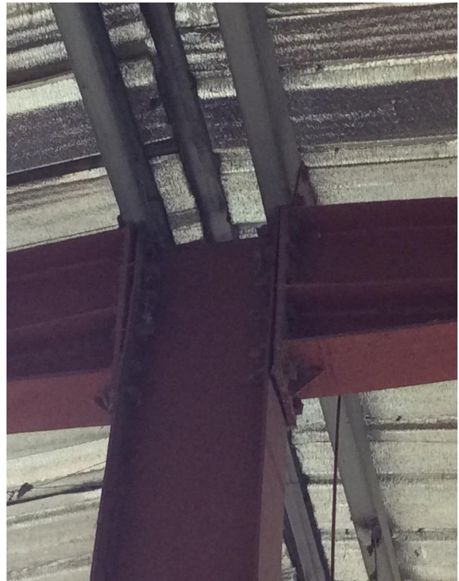
Shed 2 – Distorted end plates / inadequate bearing of end plates to central rafter support
