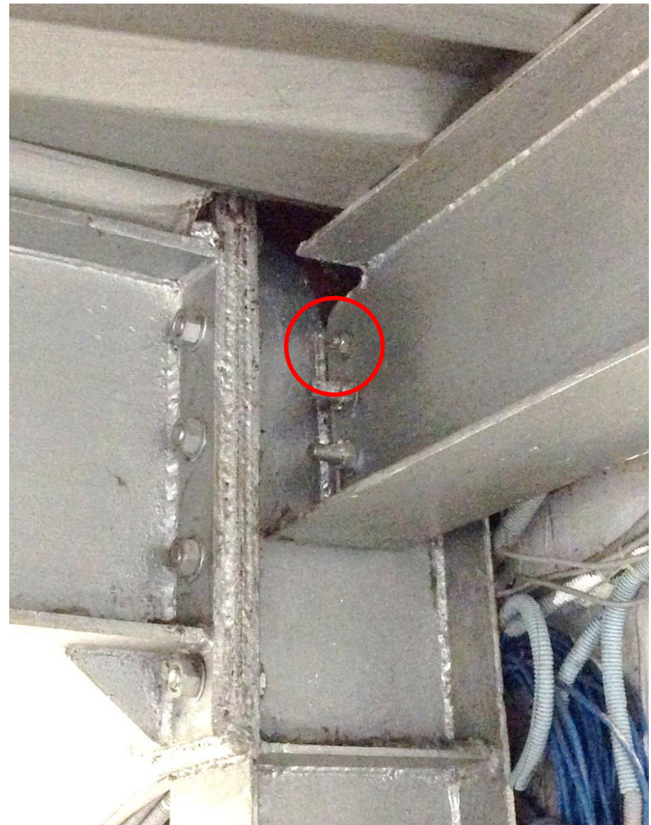
Shed 1 – Inadequate bolt replacements – it appears as though a smaller diameter bolt has been used
