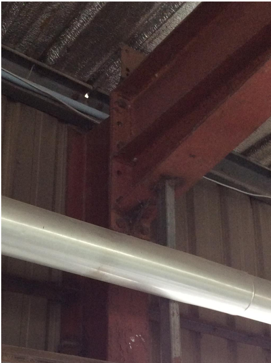
Shed 2 – Missing bolts to portal frame rafter
