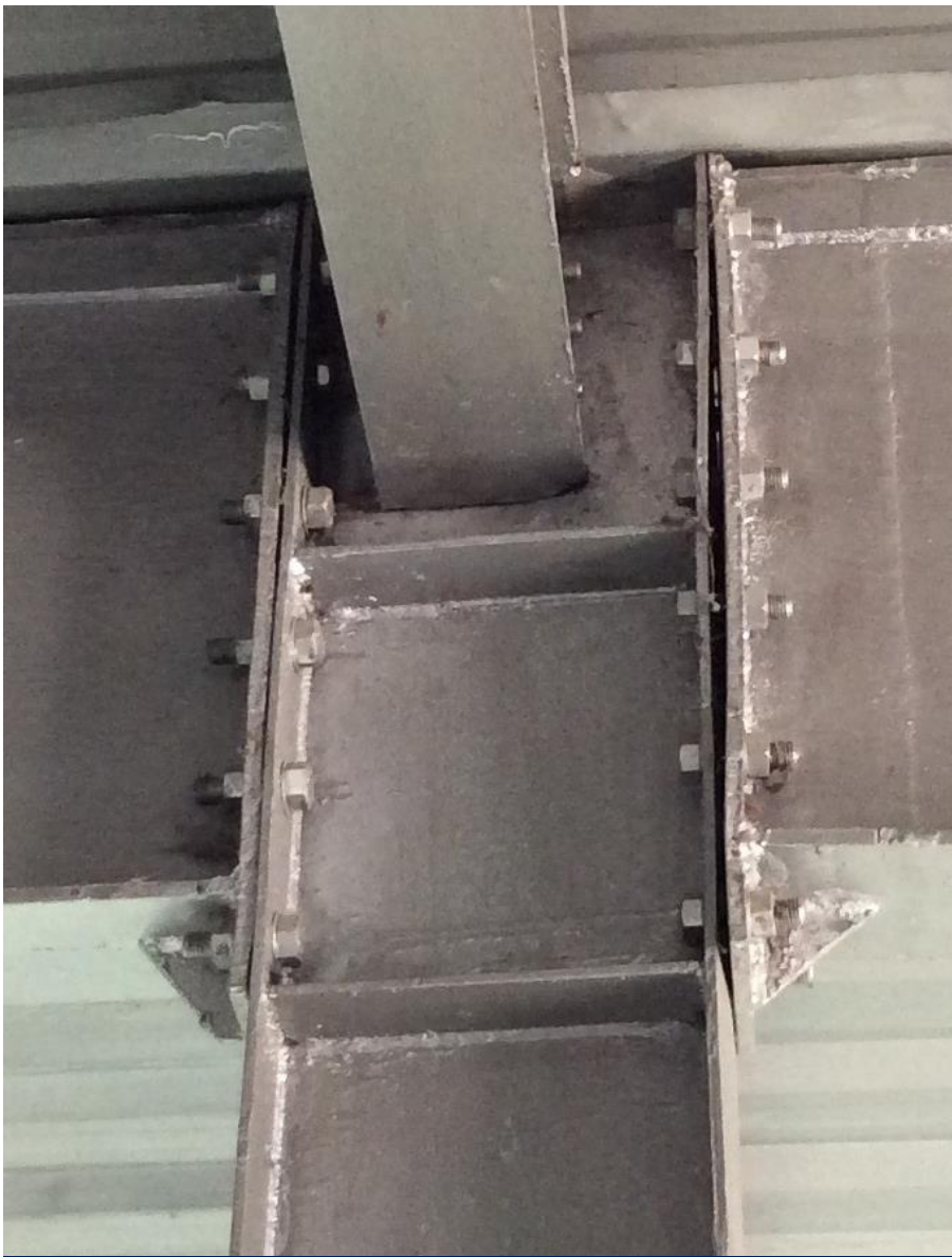
Shed 1 – Distorted end plates / inadequate bearing of end plates
