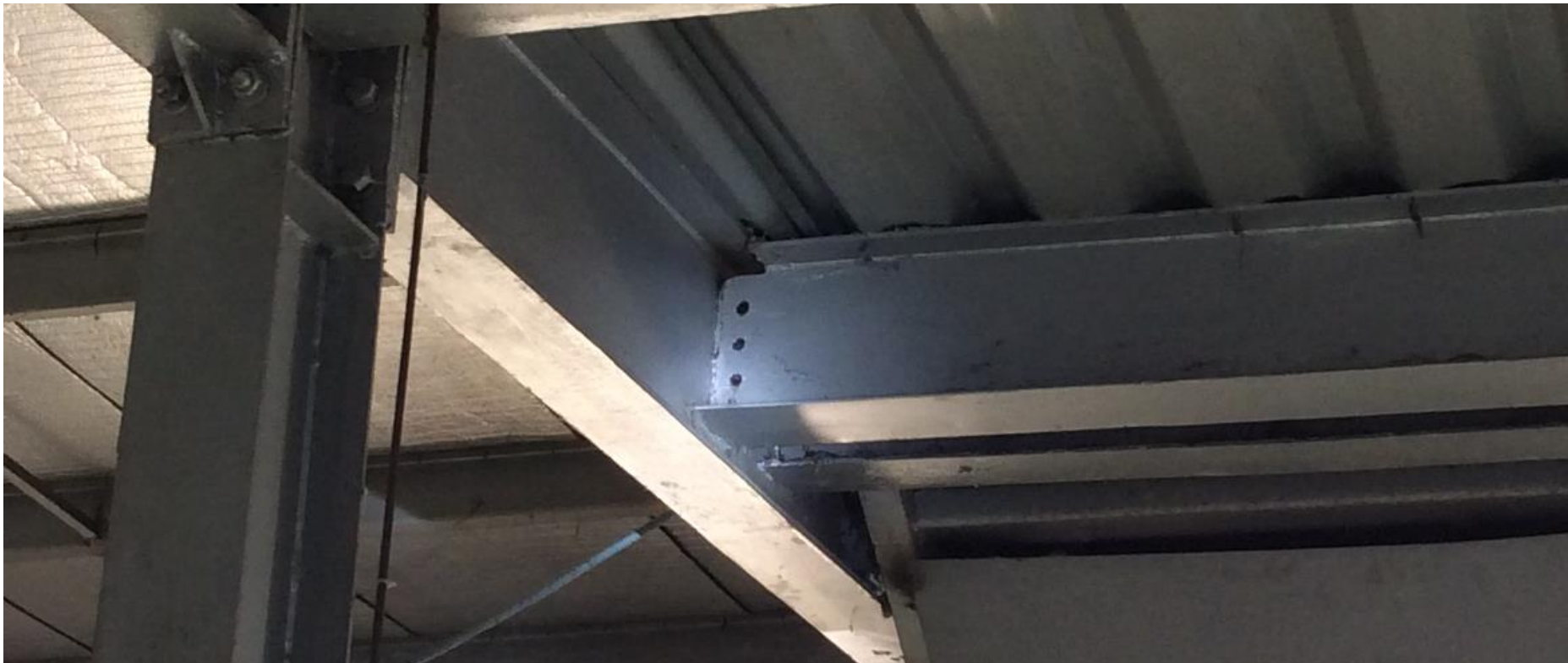
Shed 1 – Welded connection instead of bolted connection
