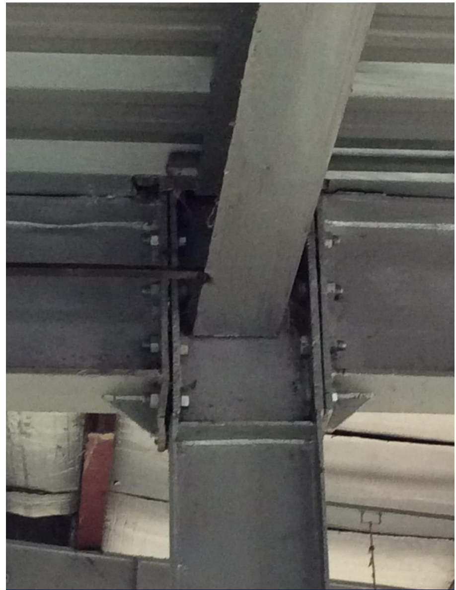
Shed 1 – Distorted end plates / inadequate bearing of end plates
