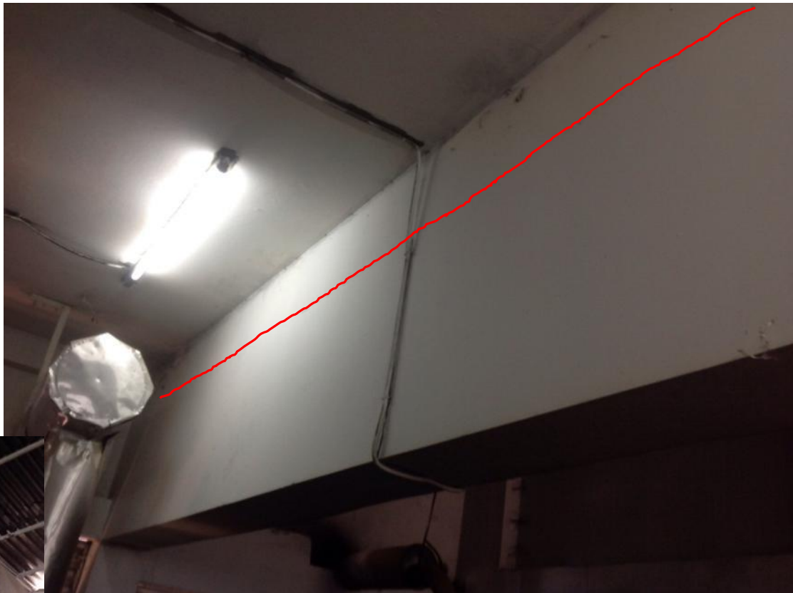
Boiler room crack along lintel
