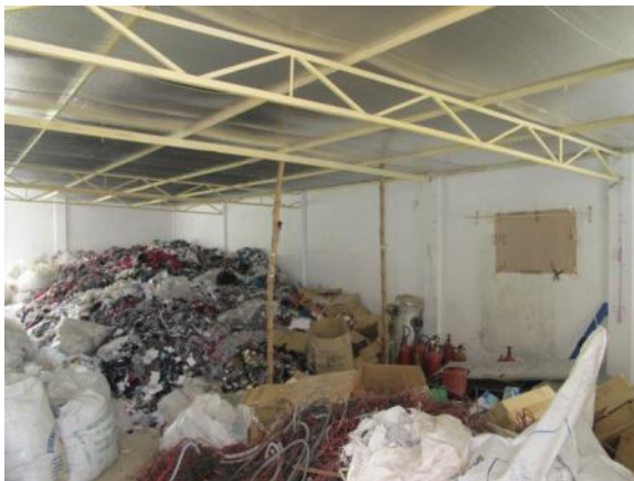
Chemical/waste storage roof structure; bamboo prop where truss missing
