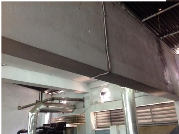
Boiler room View from other side
