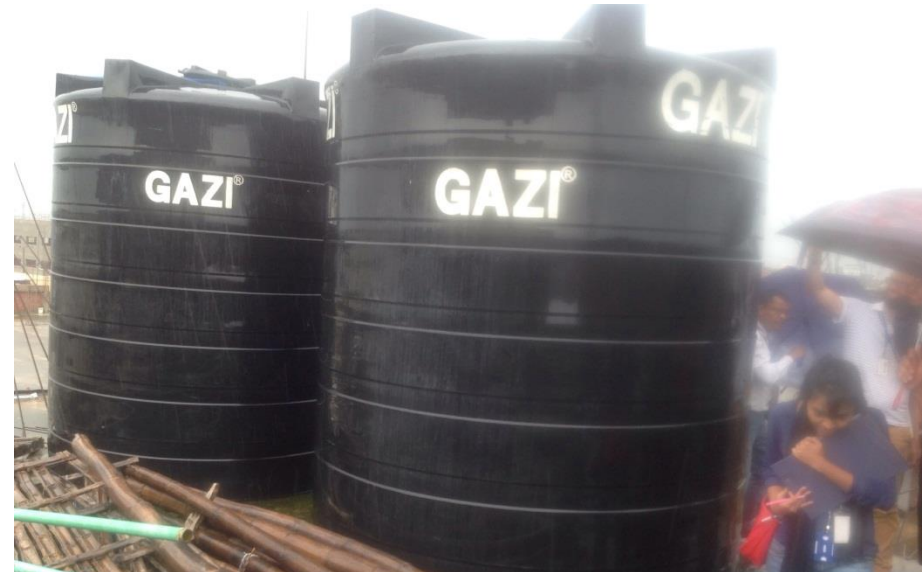
2 No. 10,000 litre water tanks on roof (2 nd Floor)
