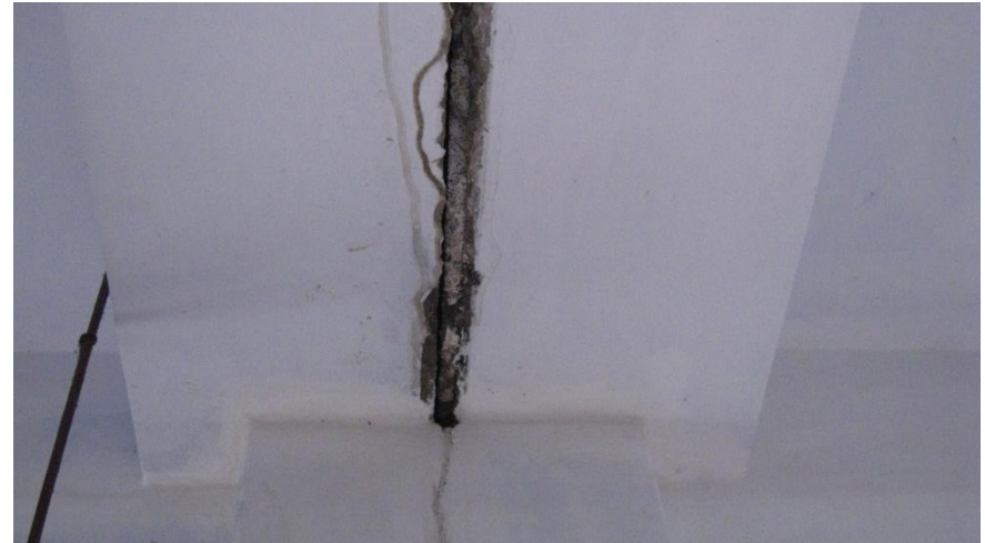
Water ingress at expansion joint
