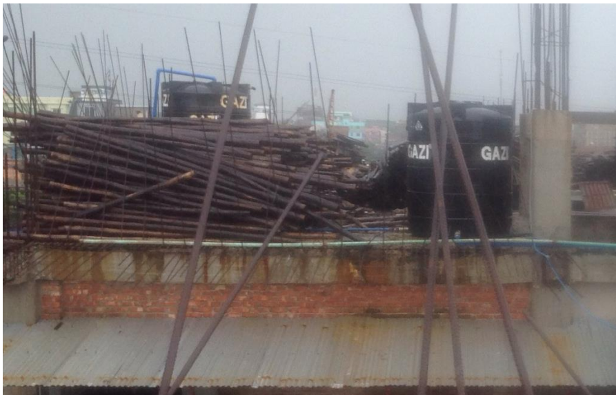
3,000 litre & 5,000 litre water tanks on roof (2 nd Floor)
