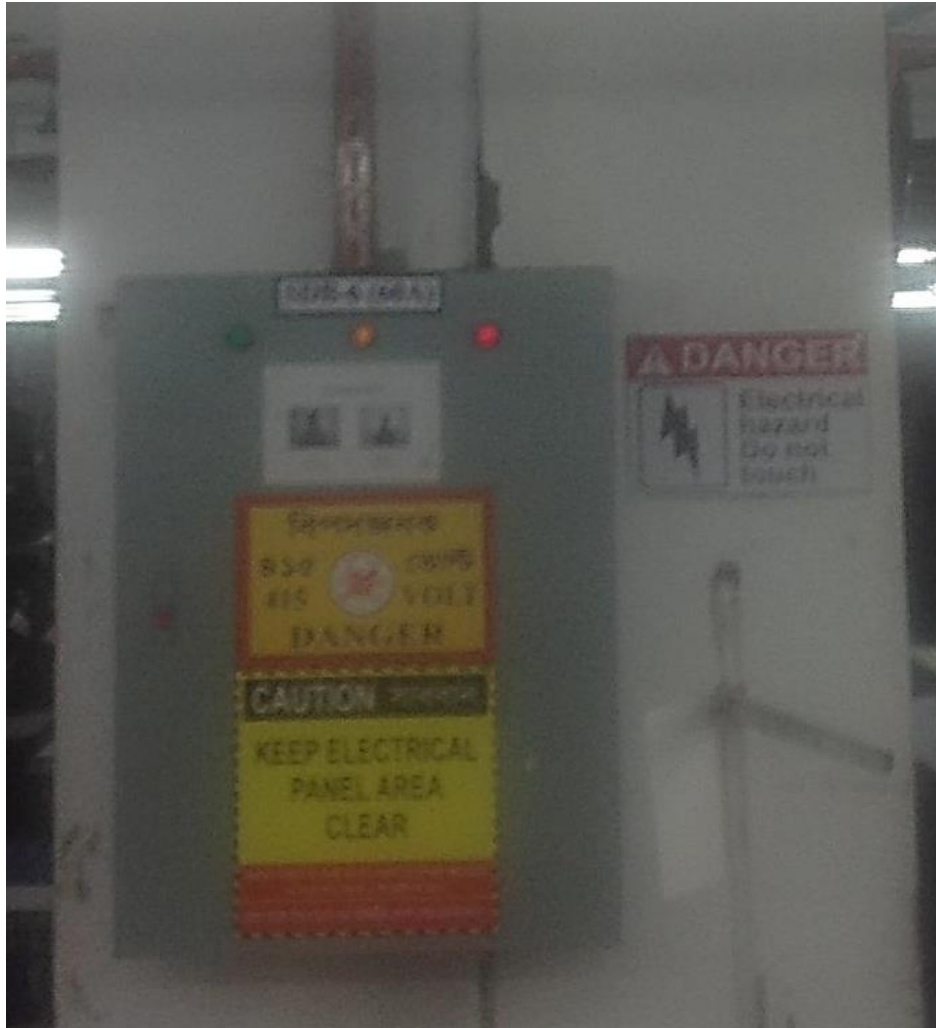
Water ingress penetrating construction joints where electrical panels are connected
