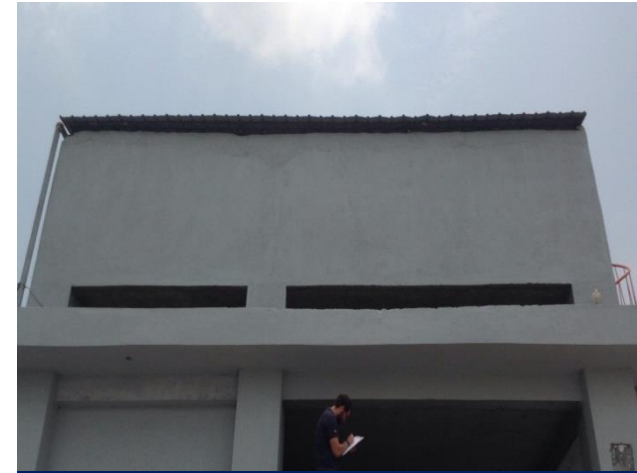
Non-engineered roof to water tank
