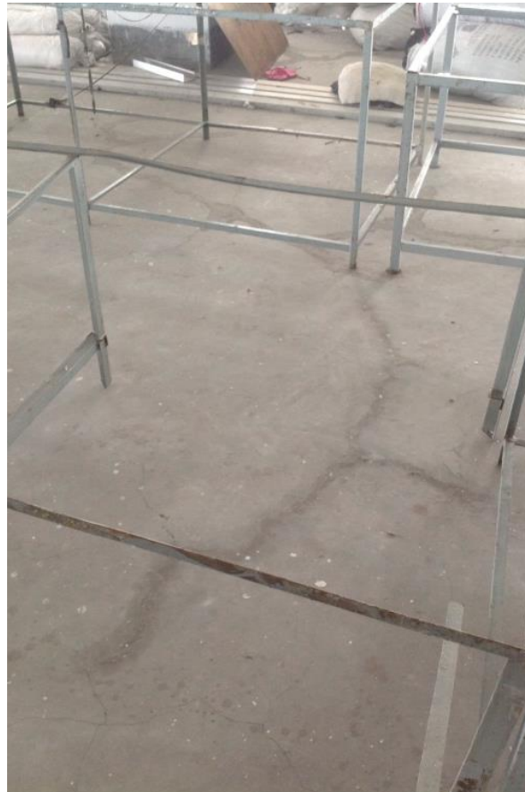
Cracking to top of slab
