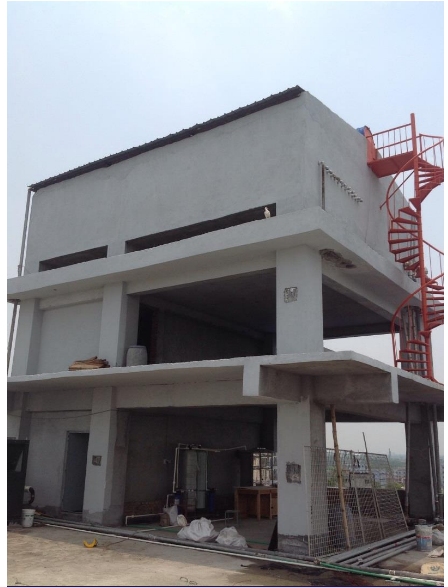
Water Tank at Roof level
