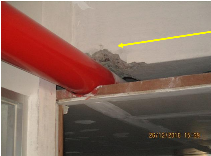
Damaged Beam at 9 th floor
