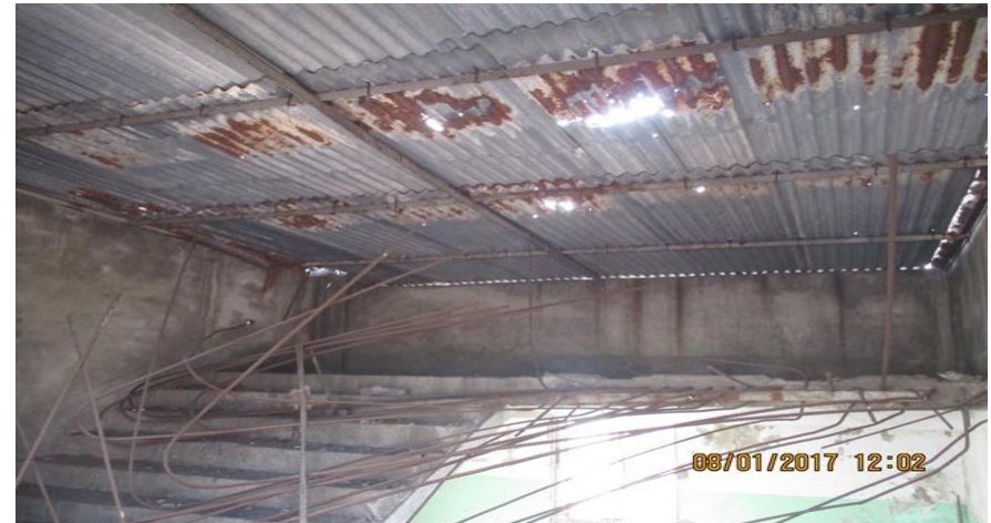
Non-engineered steel roof with corrosion
