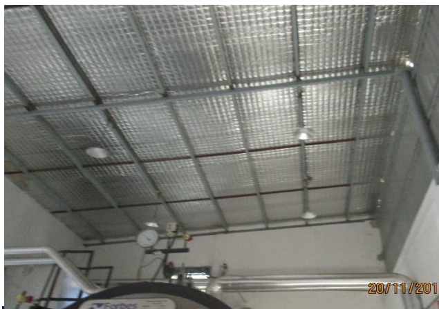
Boiler and Compressor room
