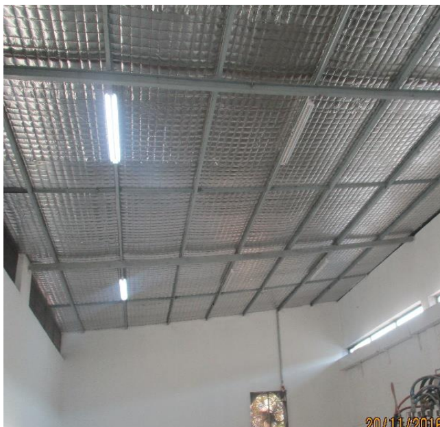
Transformer and generator room
