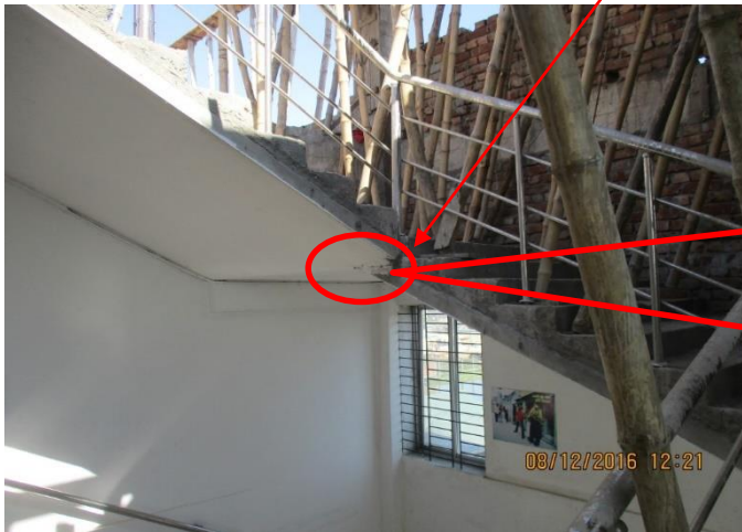
Crack on 3 rd floor waists slab of South East stair
