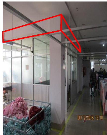
Beam was observed beside the stair case
