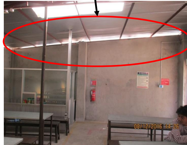
Truss was absent at both end of shed
