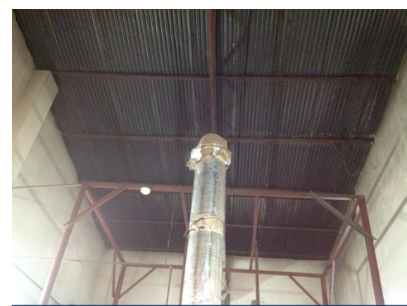
Generator & Power house
