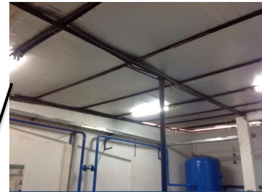
Central Compressor Unit
