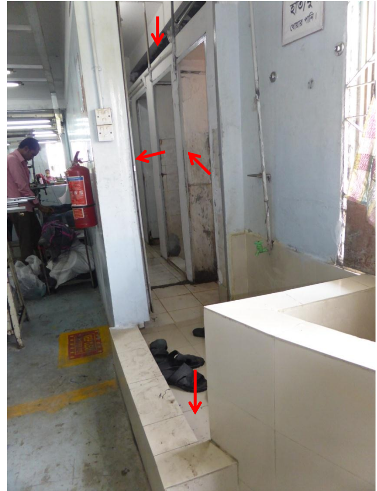
Increased floor buildup in toilet areas in addition to brick partition walls and 150mm thick concrete ceiling.
