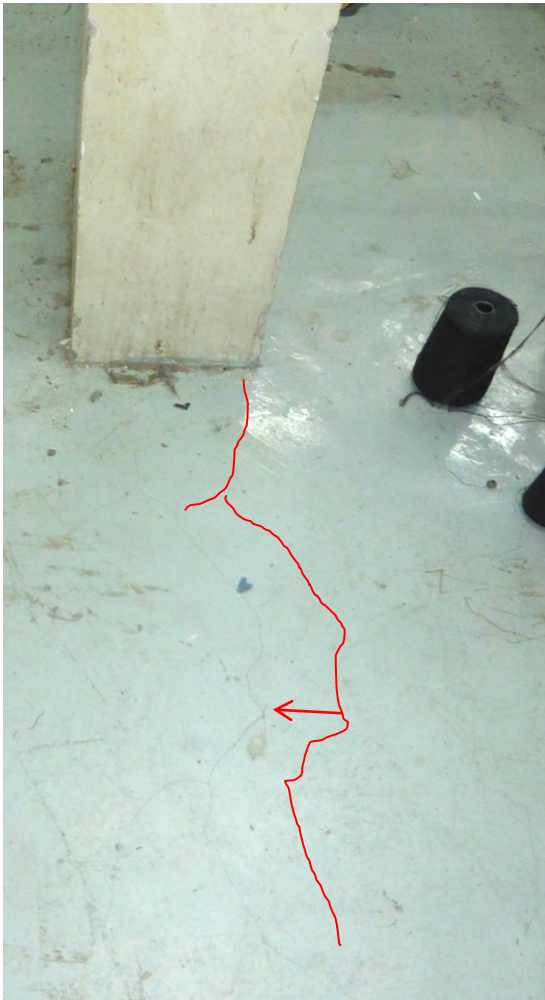
Crack above flat slab in level 4
