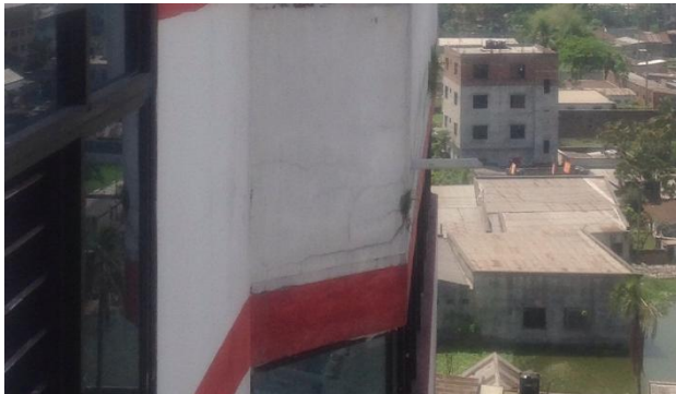
Local Cracking to Façade
