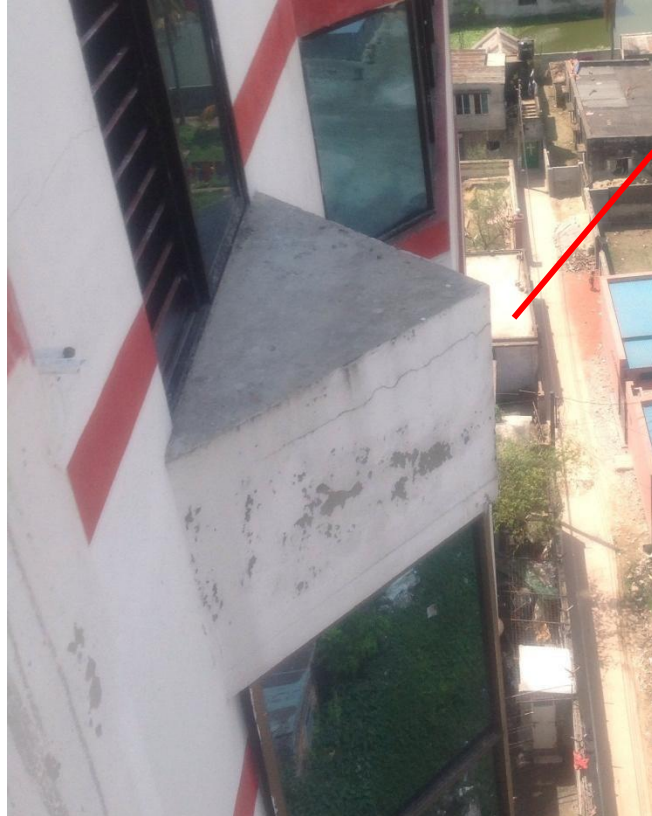
Local Cracking to Façade
