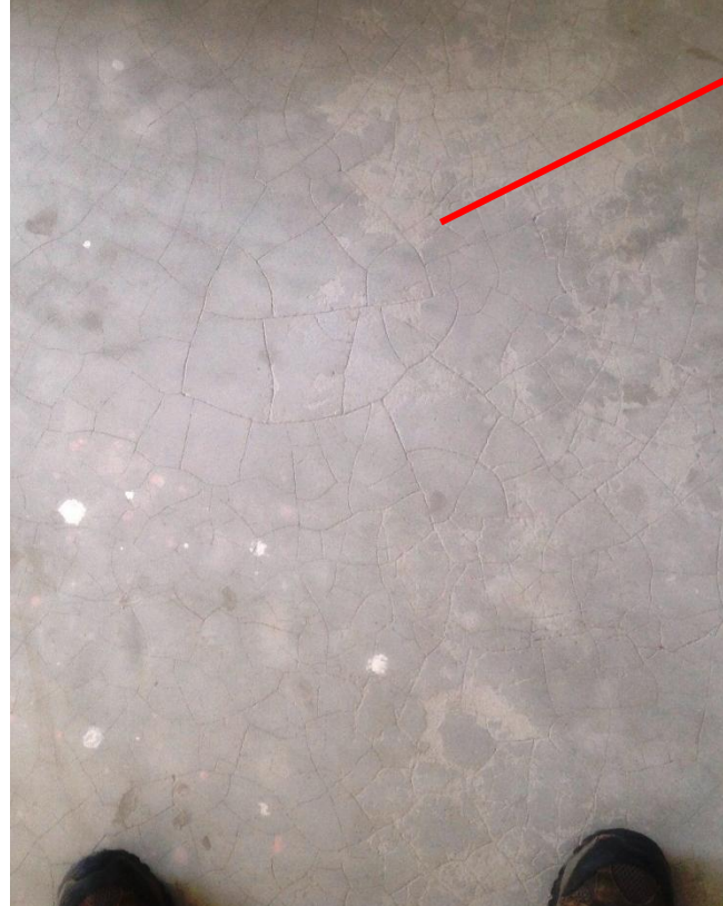
Local Cracking to 8 th Floor Slab
