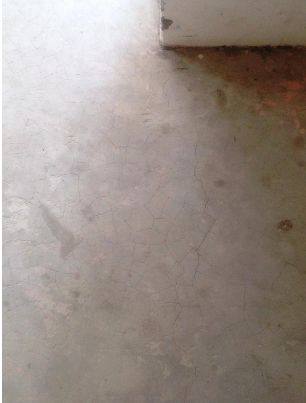
Local Cracking to 8 th Floor Slab
