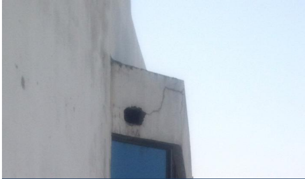
Local Cracking to Façade
