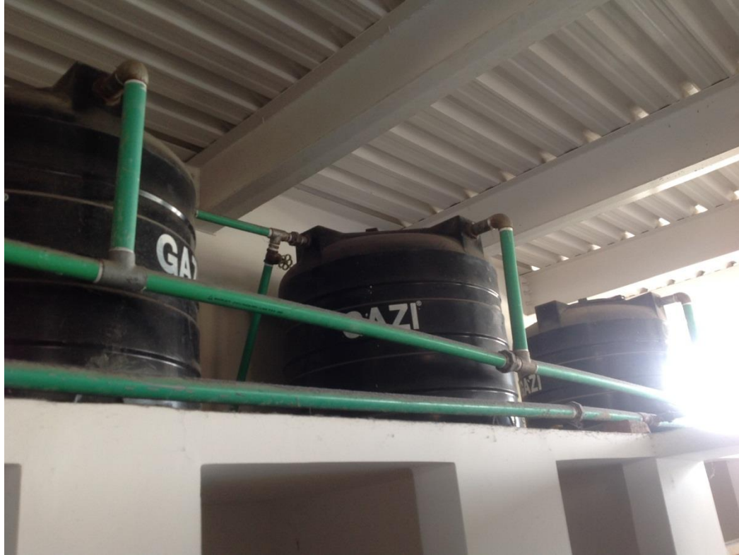
500lt water tanks over toilet ceiling
