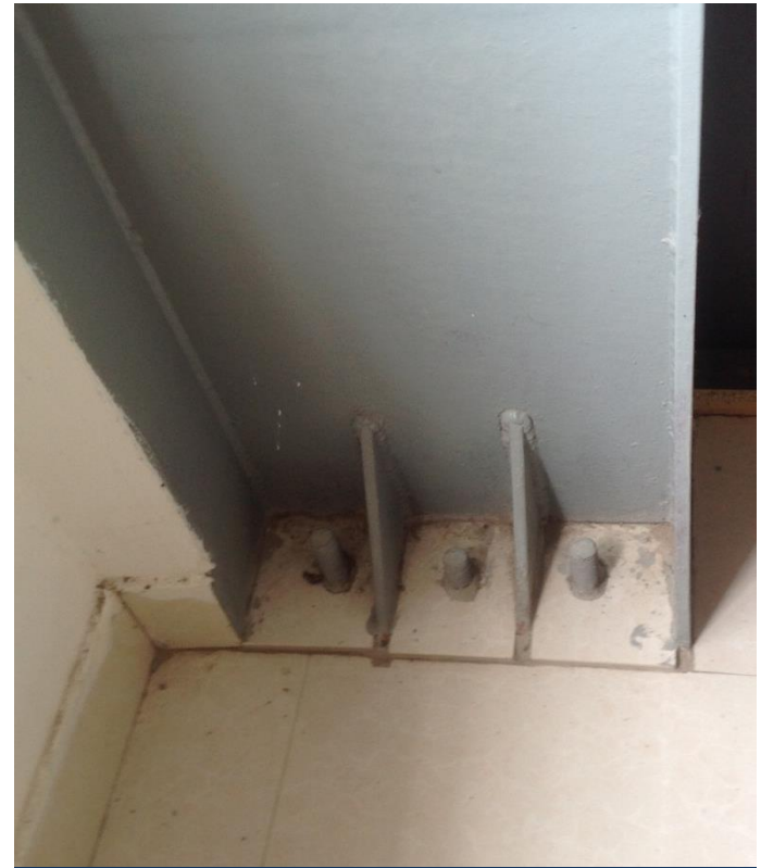
Holding down bolts missing nuts
