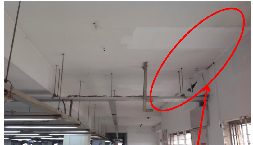
No downstand beam provided
