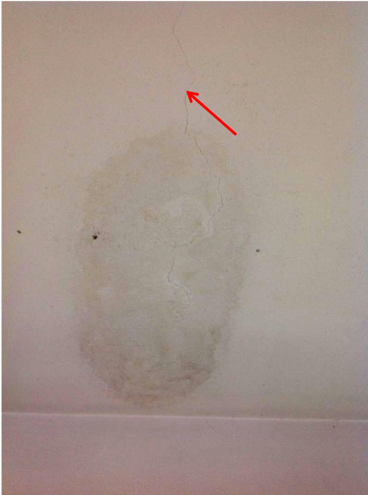
Hairline cracks observed at soffit of roof slab. Evidence of dampness in at location of crack.
