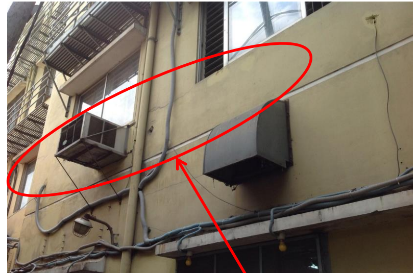
Cracking in East facade
