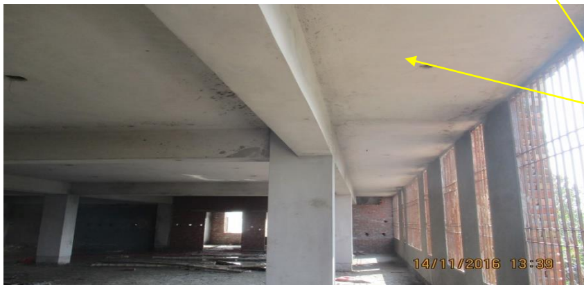
Cantilever beam missing at west side (2nd to 4 th floor)
