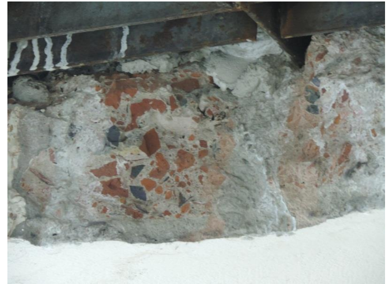
Brick aggregate in floor slab
