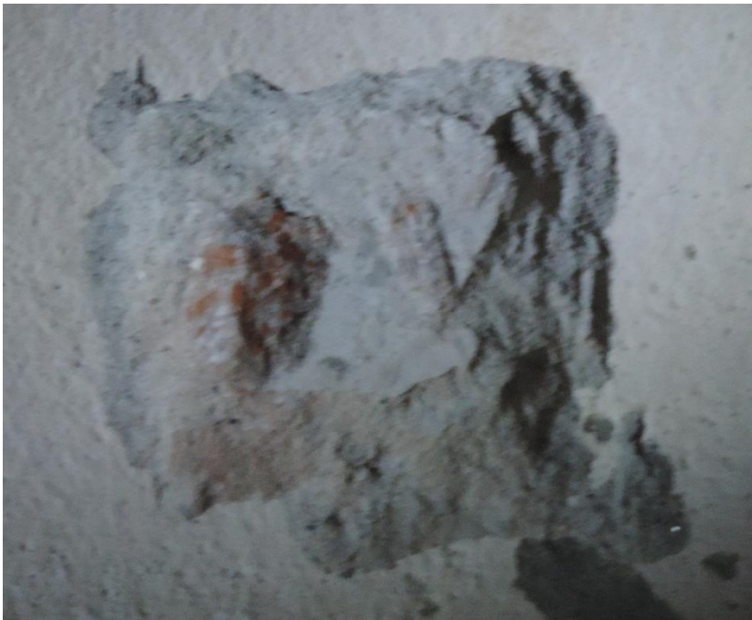
Brick aggregate in Ground Floor column
