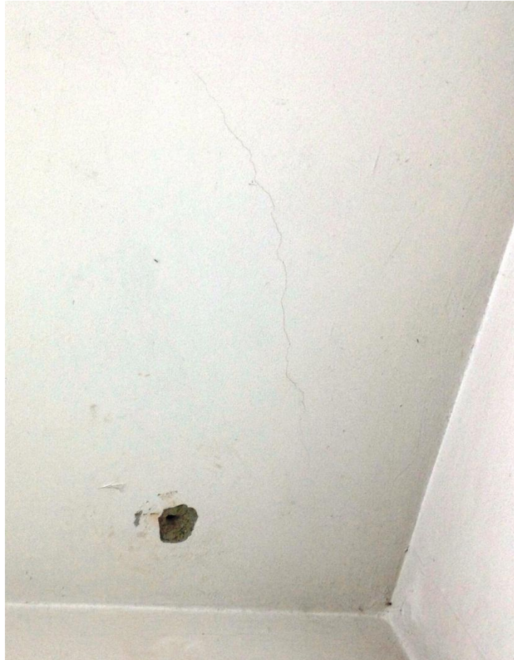
Cracking to underside of 5 th Floor slab
