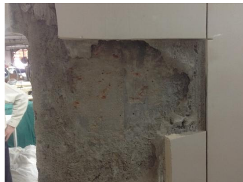
Tested Column D/3 (Brick)
