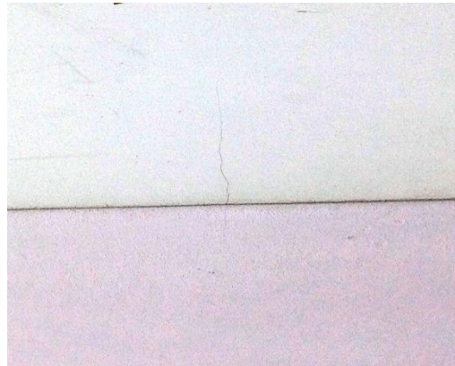
Cracking to 2 nd Floor beam
