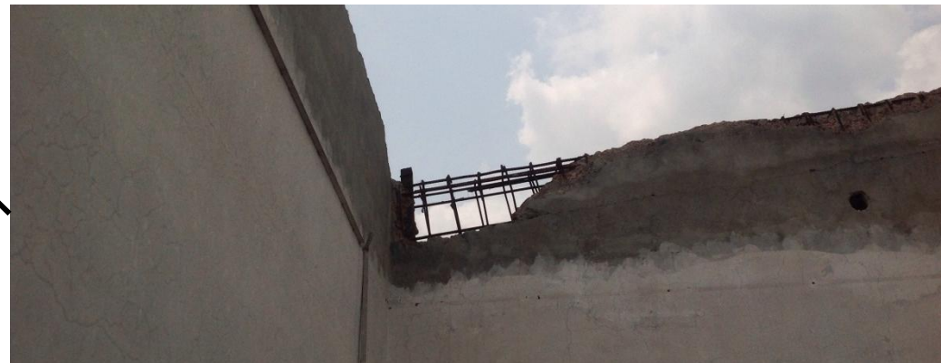
Exposed reinforcement to section of gable-end ring beam
