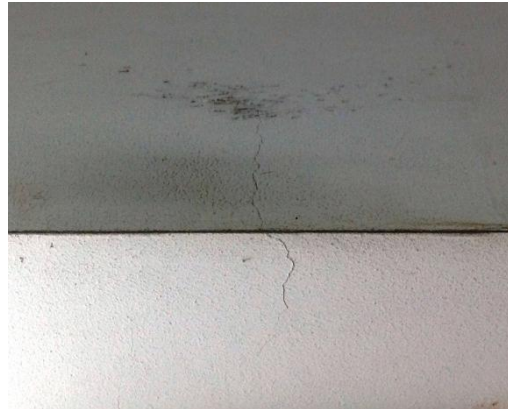
Cracking to 5 th Floor beam
