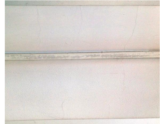
Cracking to 3 rd Floor beam
