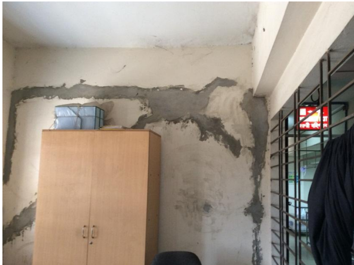
Cracking in internal brickwork wall
