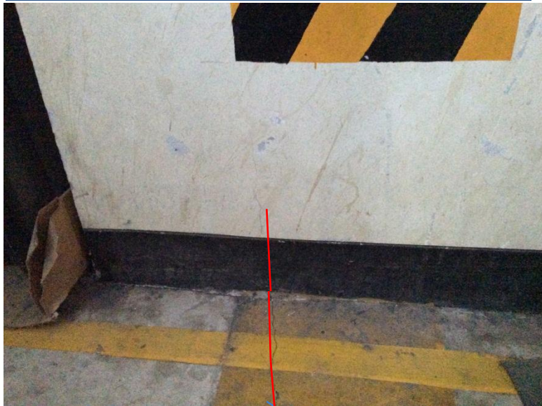
Cracking on ground floor adjacent to column
