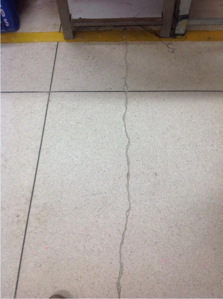
Multiple cracking in floor finish.
