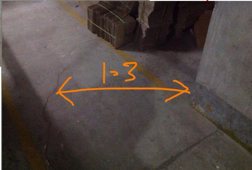
Cracking in basement slab
