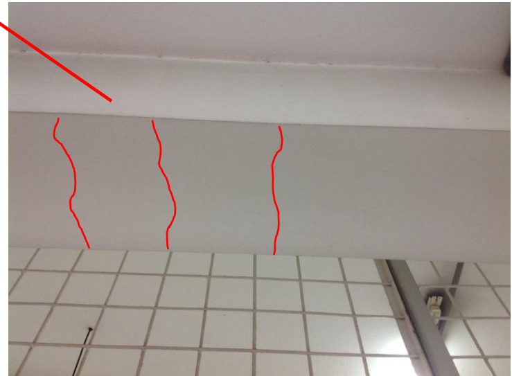
Cracking in beam supporting 2 nd floor
