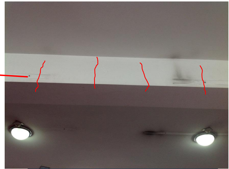
Cracking in beam supporting 5 th floor
