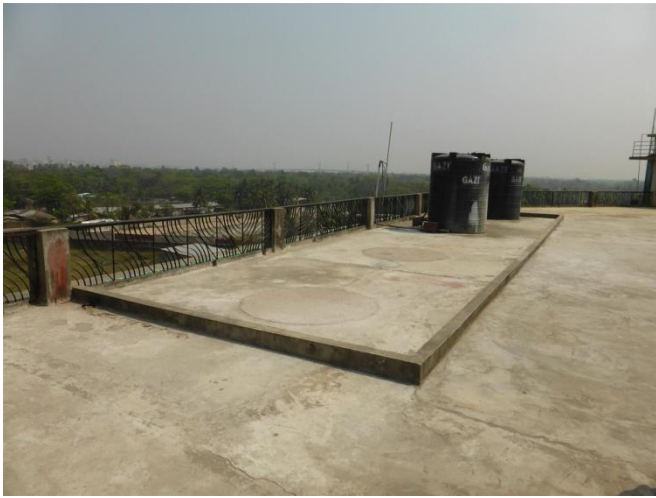
Water tanks at roof level
