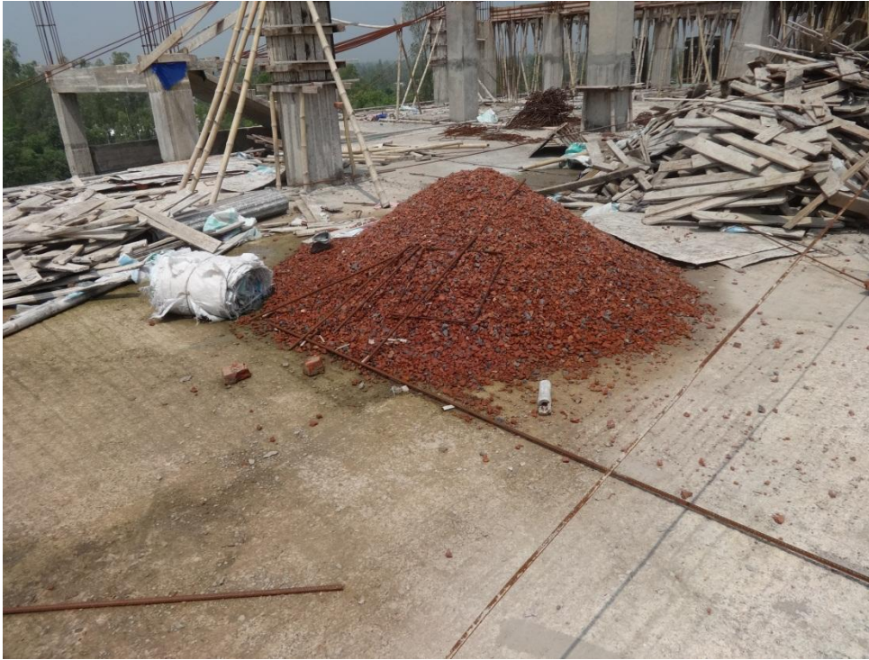
Brick aggregate and other construction materials stored on present fifth floor (roof).
