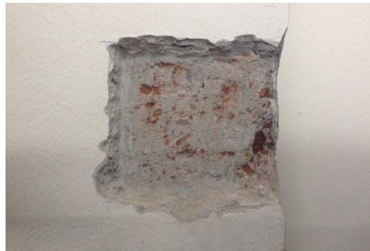
Tested Column D/5 (Brick)
