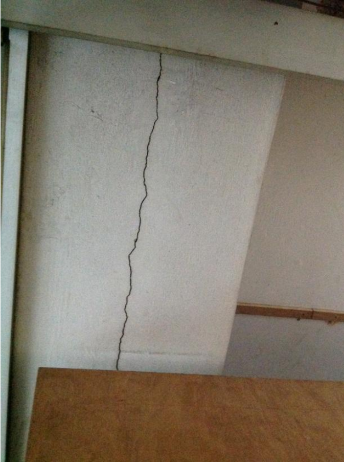
Cracking in beam
