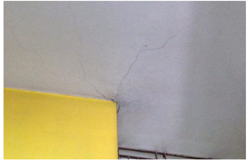
Cracking in slab
