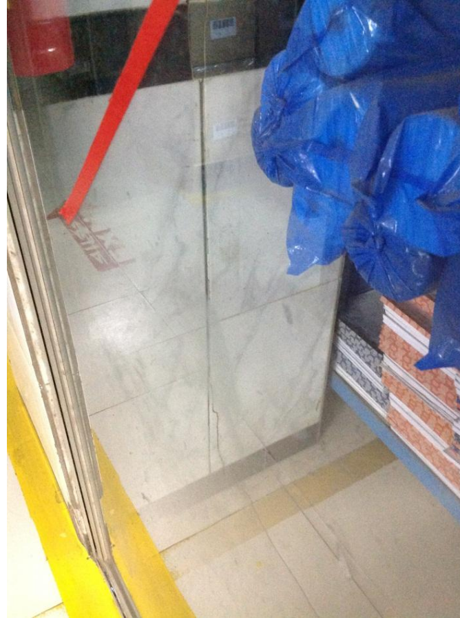
Cracking in slab
