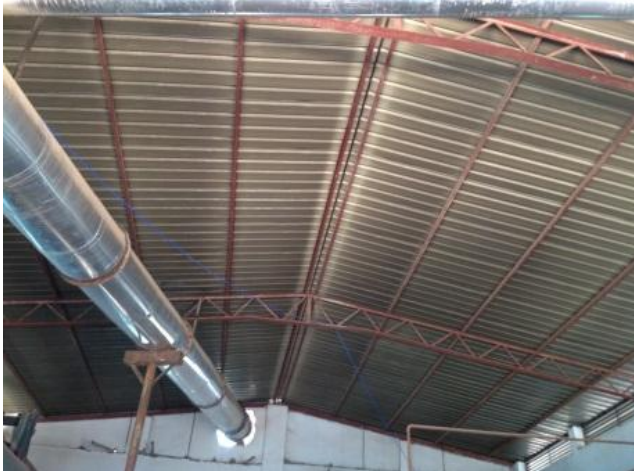
Lack of roof bracing
